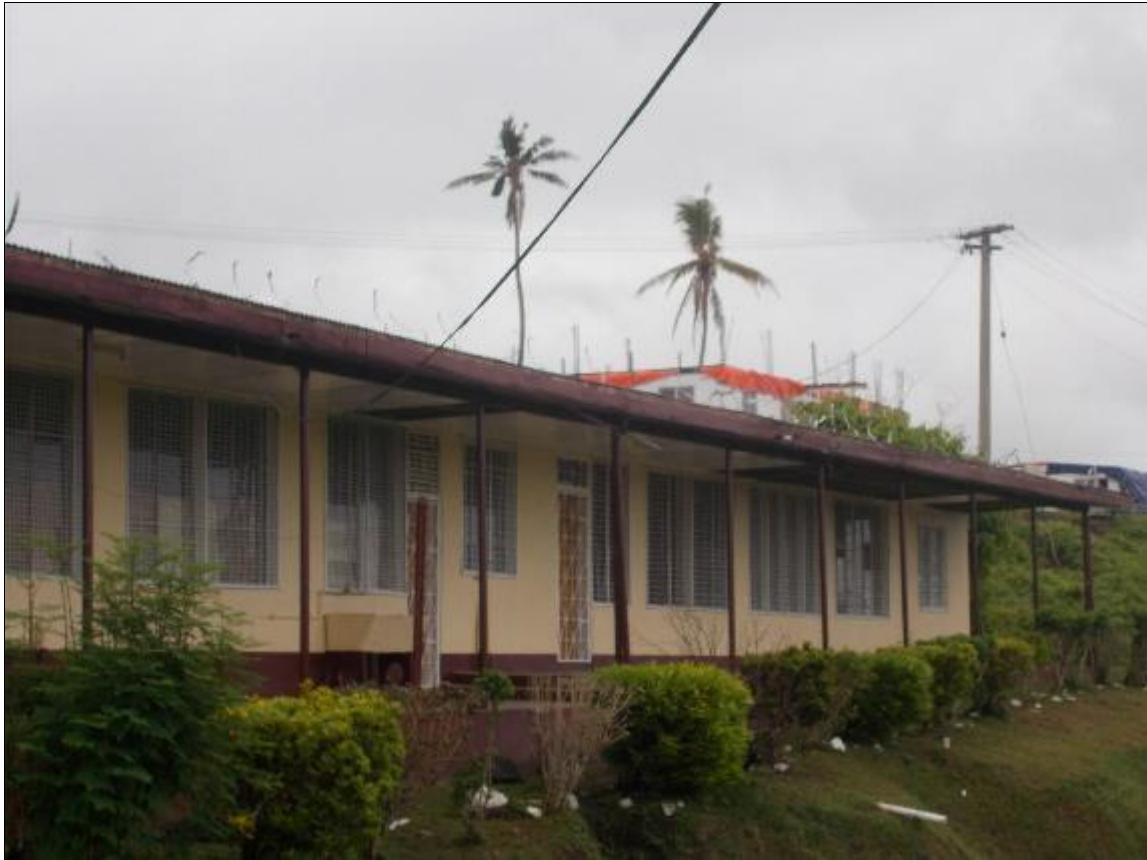
Photo 3: Showing Gutter Damaged/Blown Away
