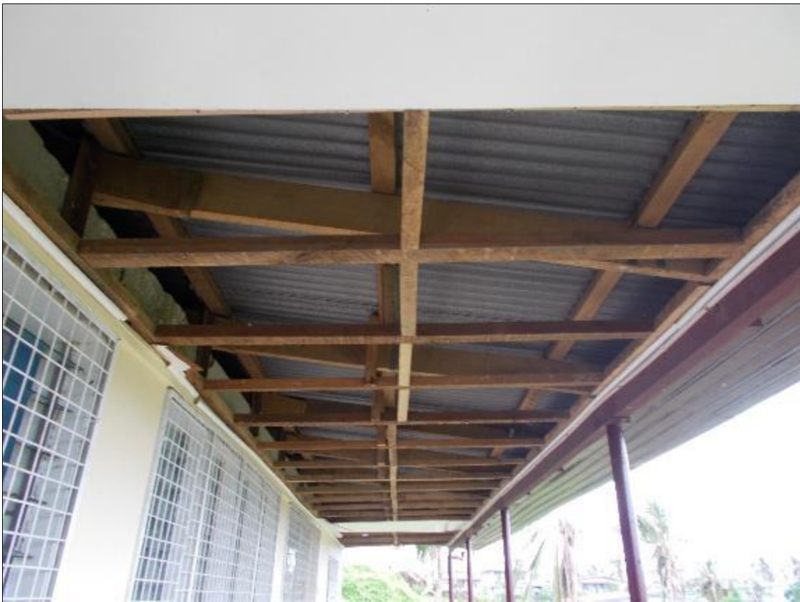
Photo 4: Showing Verandah Ceiling Damaged/ Blown away
