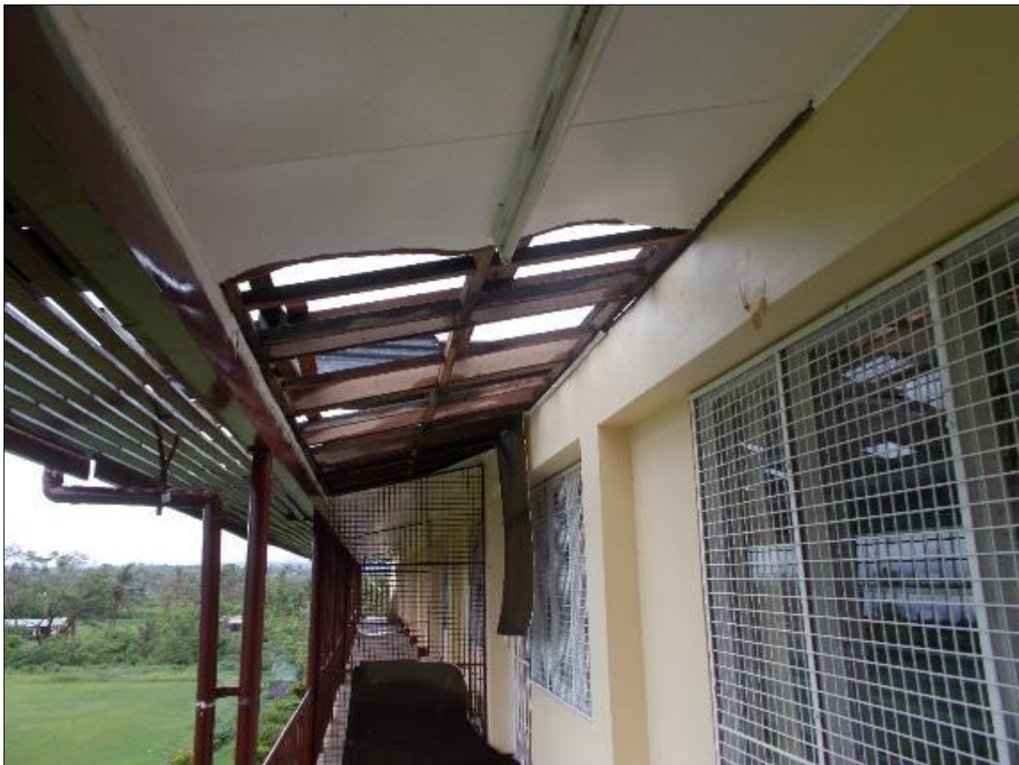
Photo 8: Verandah Ceiling Damaged/ Blown away
