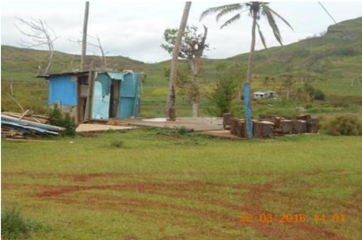
Photo 12:View of the Damaged Teachers Quarters
