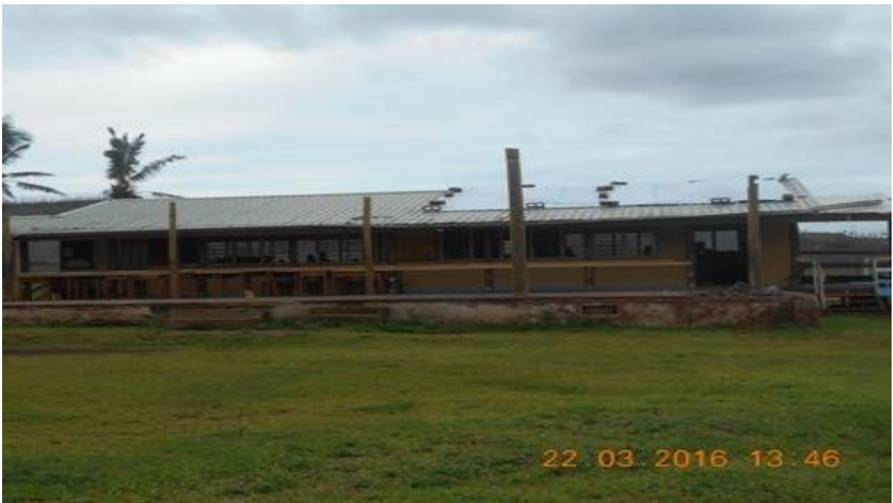
Photo 2: View of Damaged School Building
