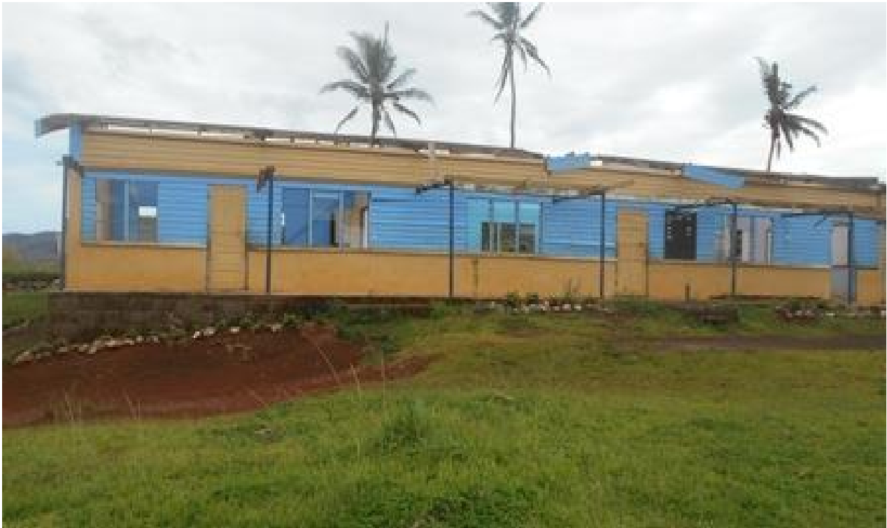
Photo 1:View of the Damaged School Block
