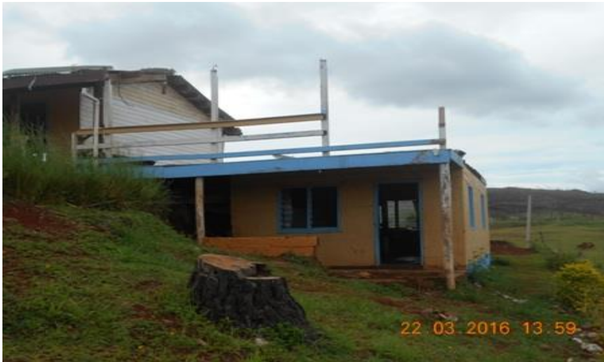
Photo 3: View of Damaged School Basement
