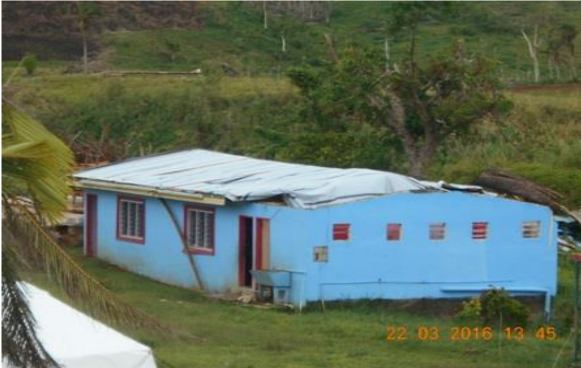
Photo 6: View of the Damaged Boys Dormitory
