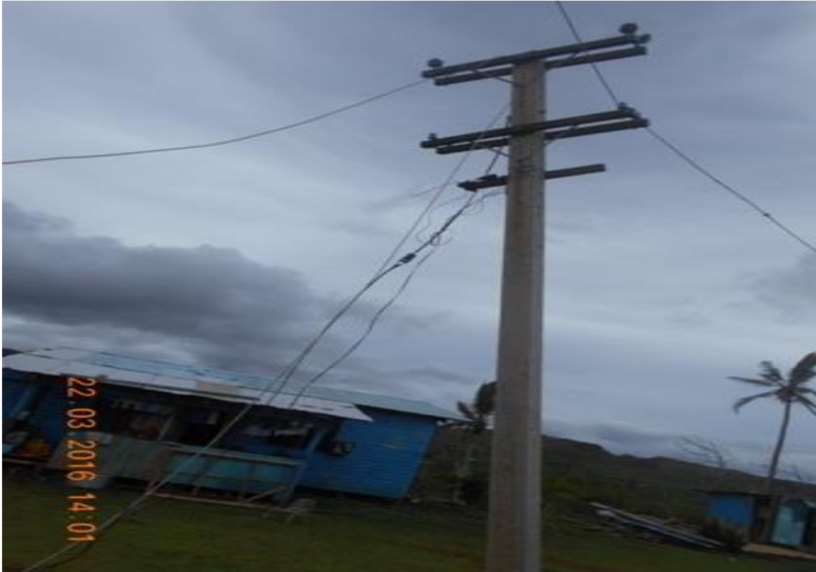
Photo 13: View of Damaged FEA Post and Electric Cables
