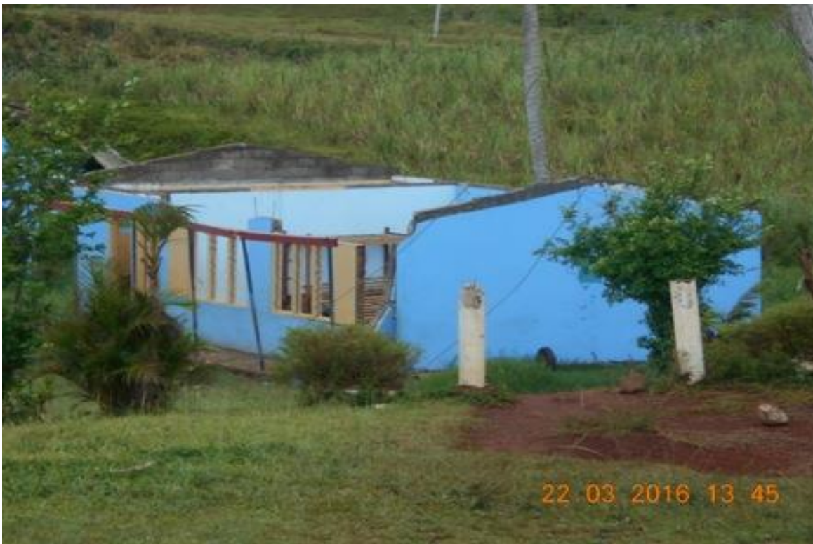
Photo 7: View of the Damaged Girls Dormitory
