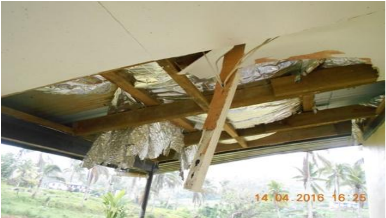
Photo 1: Portion of roof damaged with ceiling
