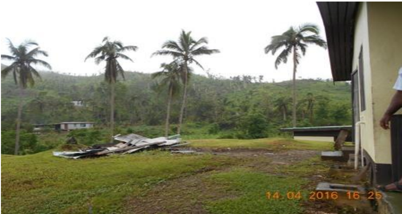
Photo 2: Kitchen Portion of Dining been blown away
