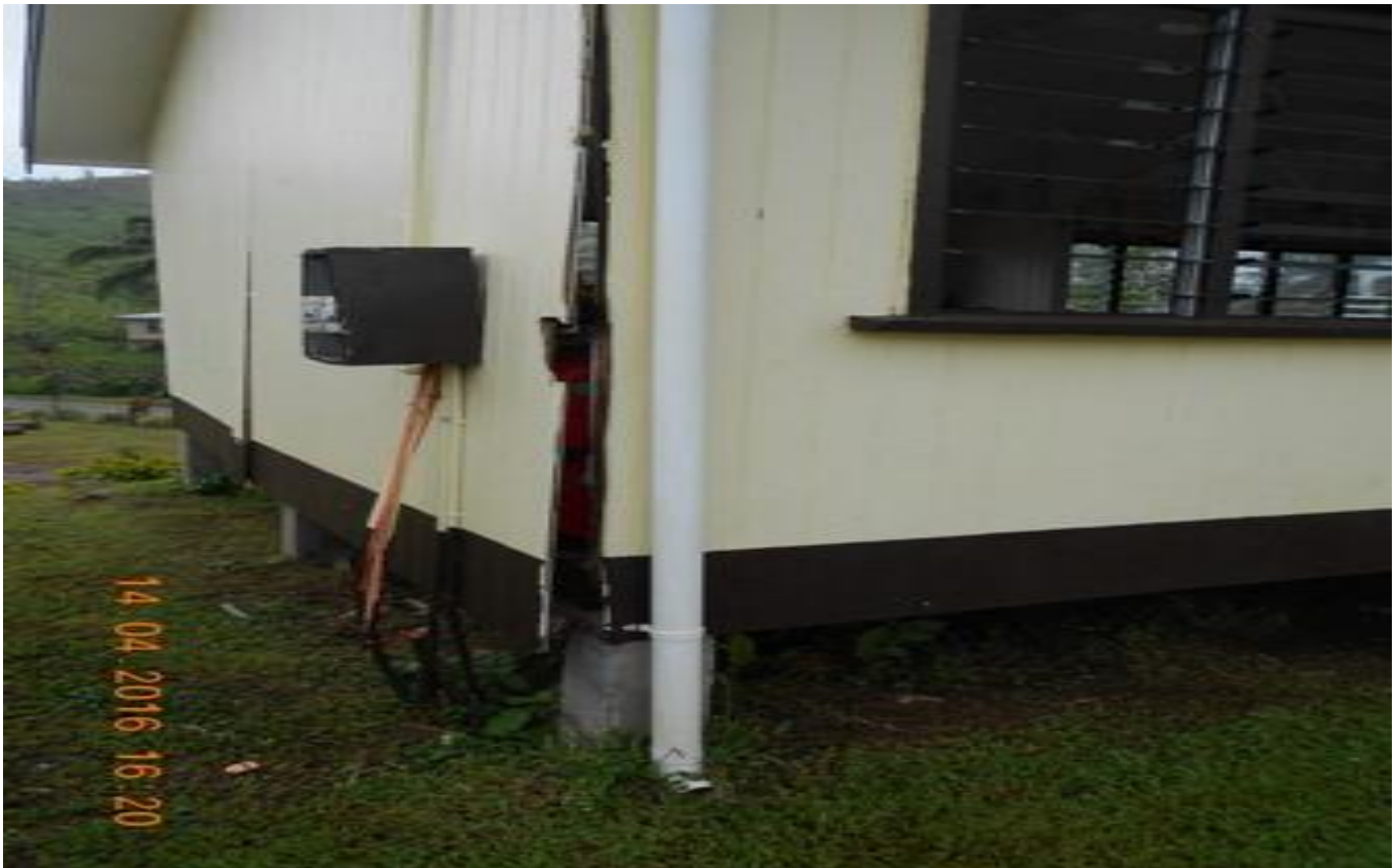
Photo 4: Damaged Gutters & Down pipes
