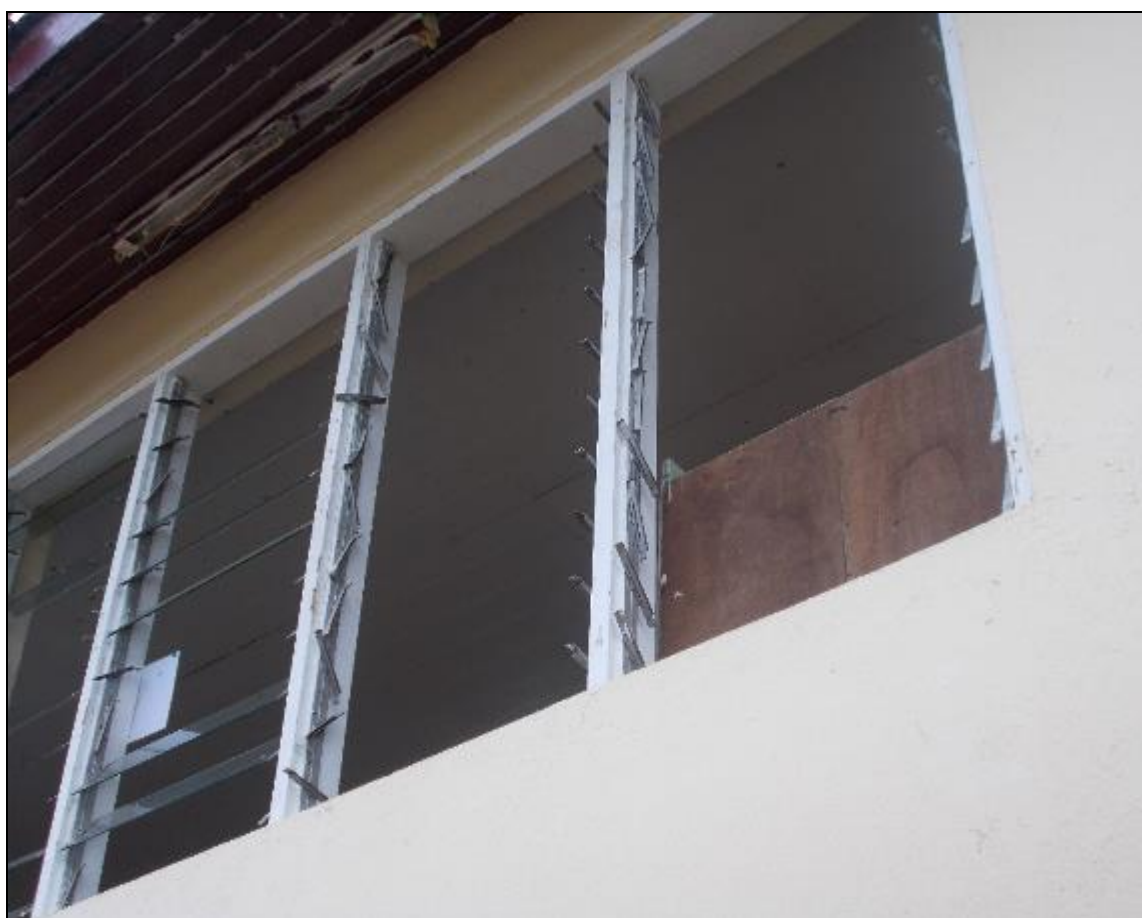
Photo 4: View of damaged louver blades
