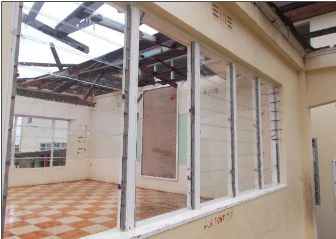
Photo 9: Damaged louver blades/ roof frame.
