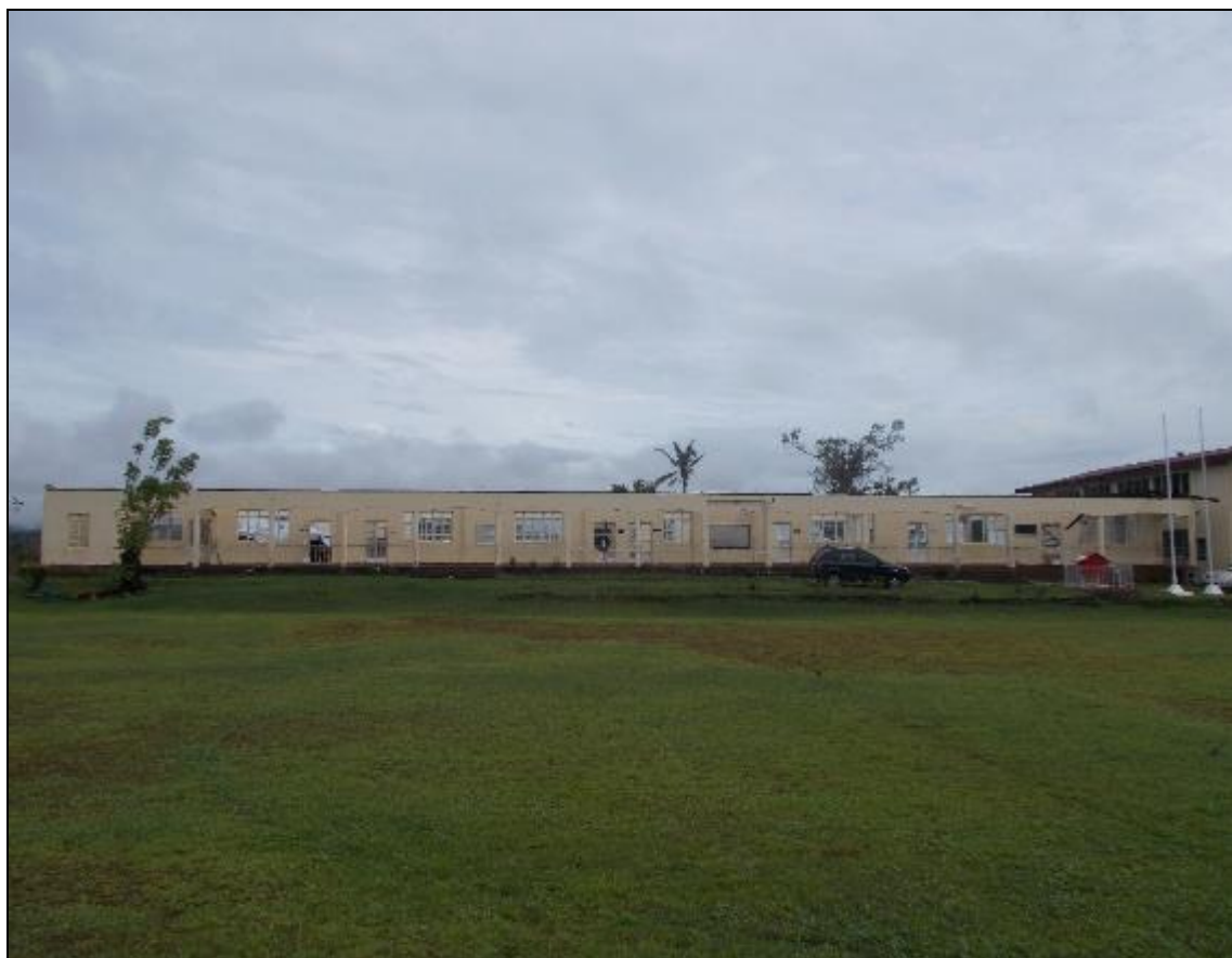
Photo 6: Overall Side View of Block B- Blown off roof
