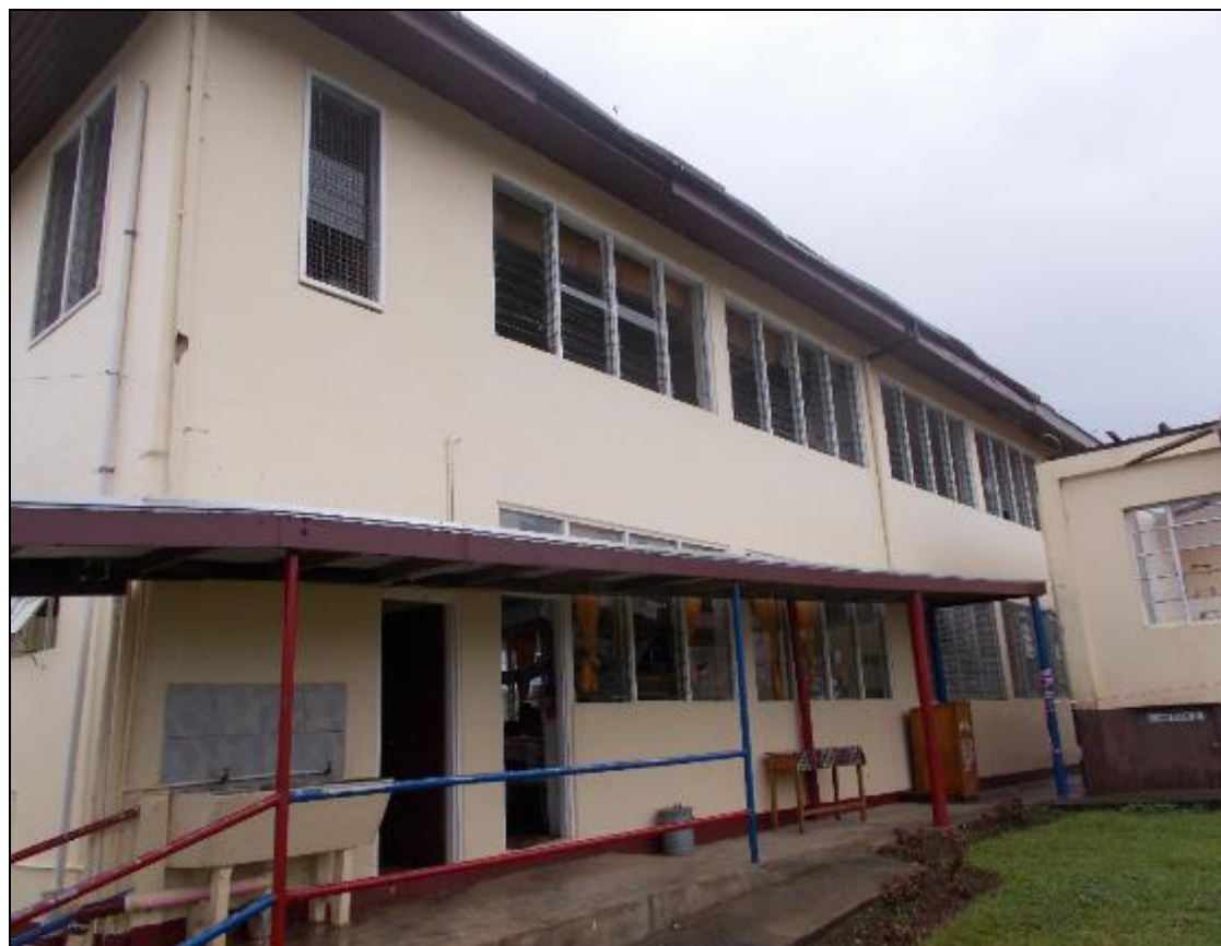
Photo 2: Rear view of Block A- Damaged Gutter.
