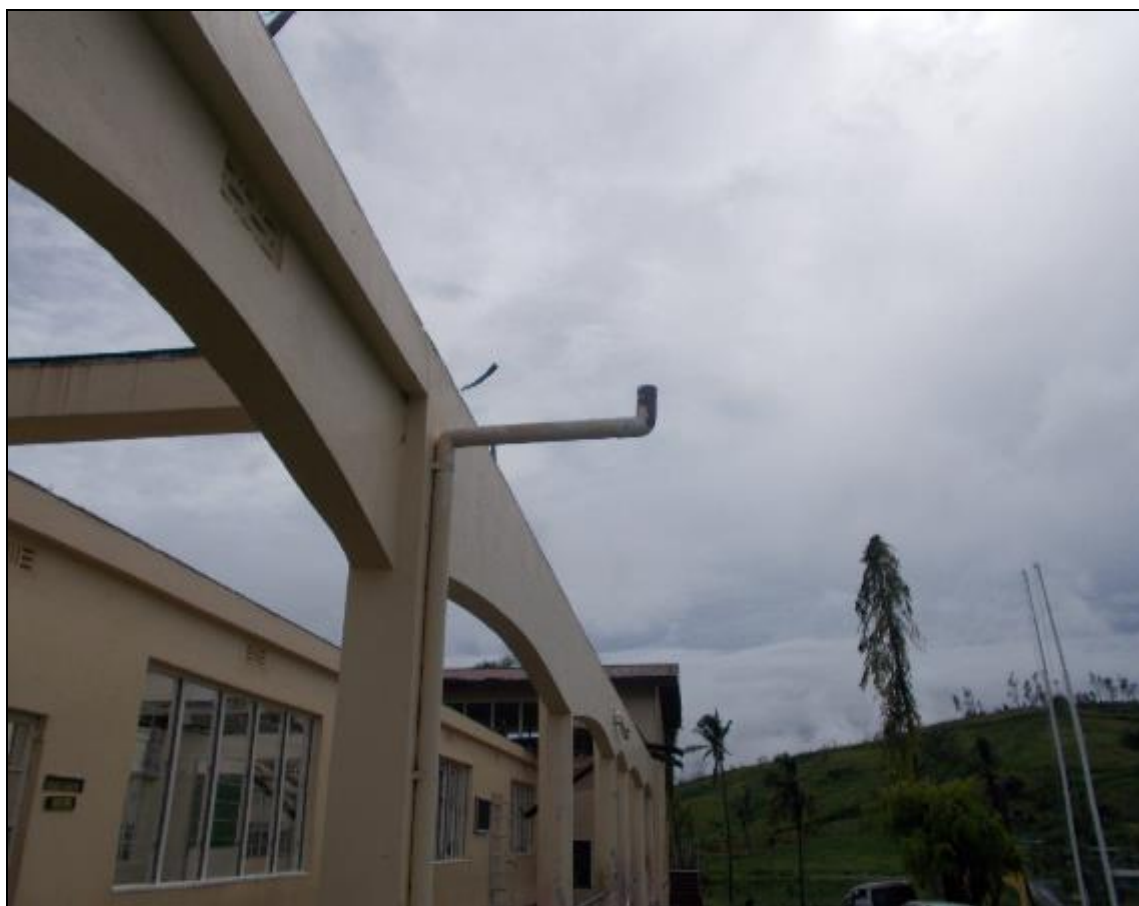
Photo 12: Damaged down pipe, blown off fascia boards and gutters
