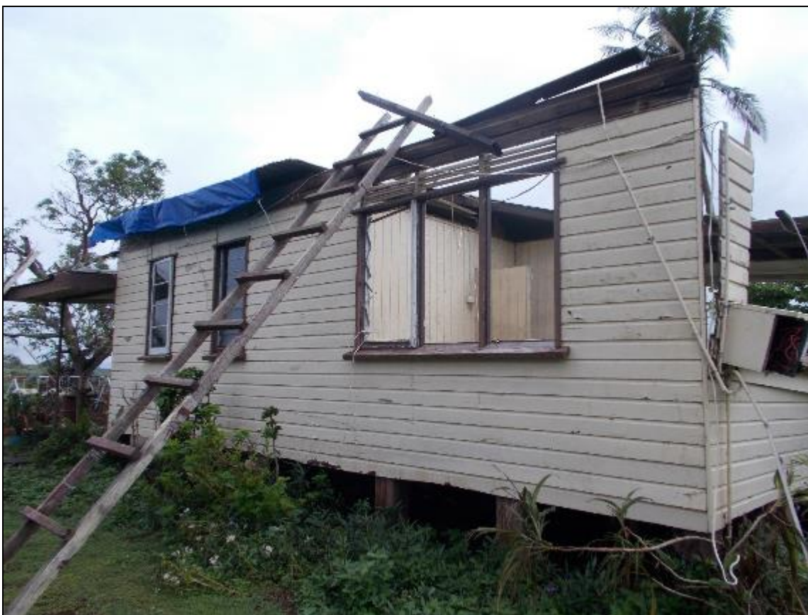
Photo 15: Side view of damaged Staff Quarters 1- Damaged gutters,downpipes,walls,etc.
