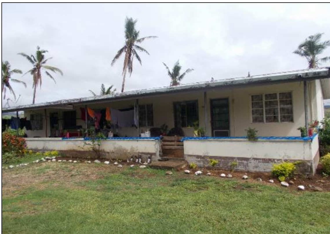
Photo 16: Front view of damaged Staff Quarters 2- Damaged and warped gutters
