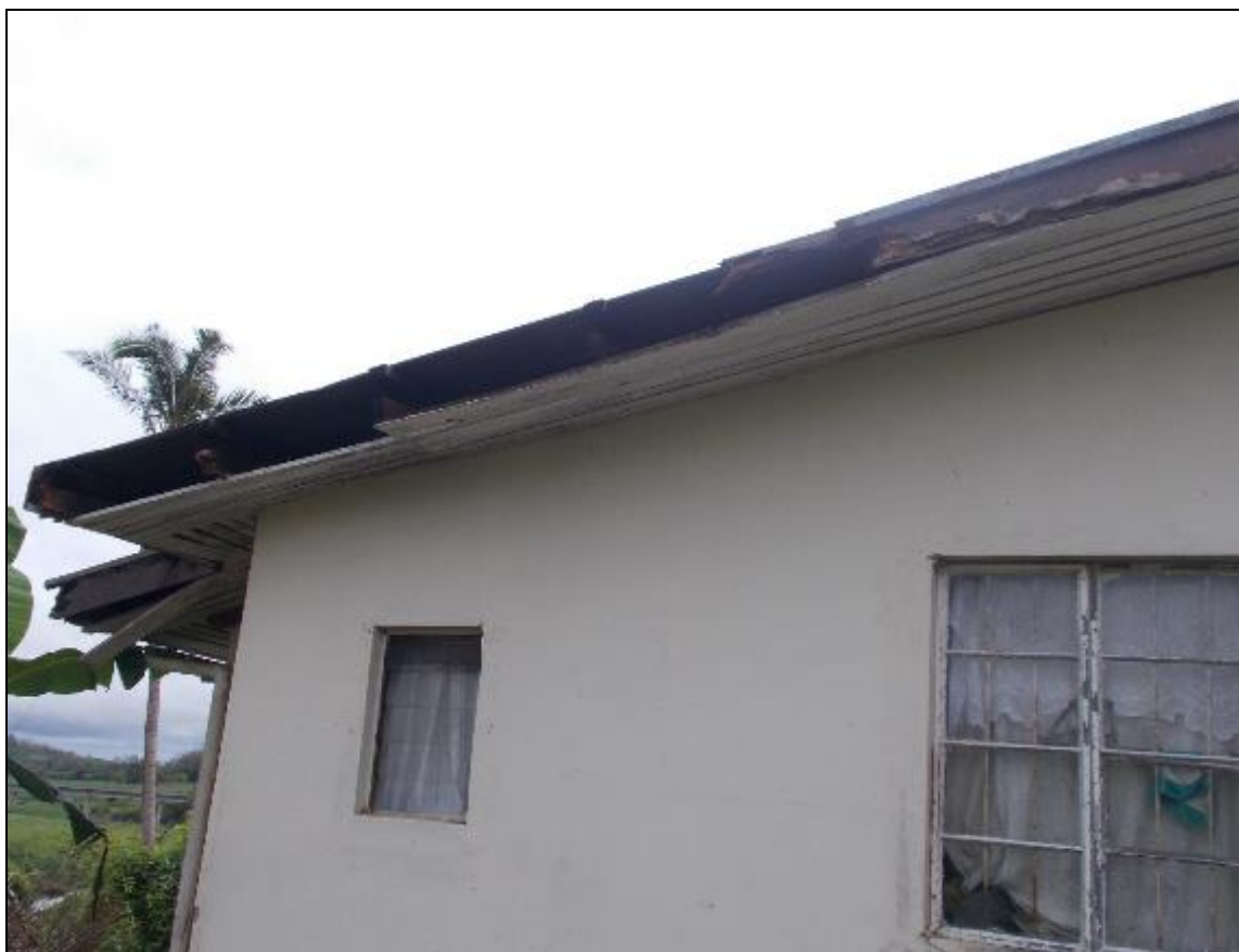
Photo 17: Damaged Fascia Board.
