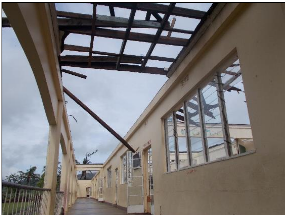
Photo 13: View of damaged verandah area
