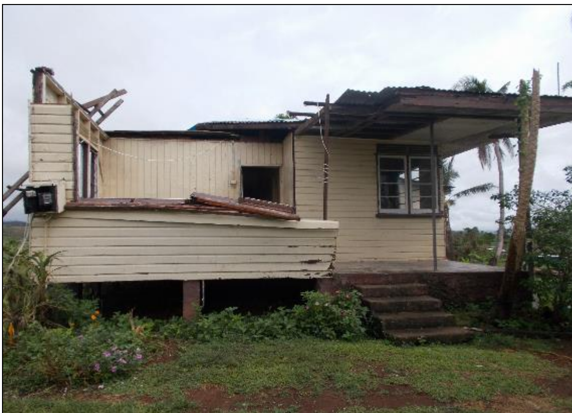
Photo 14: Front view of damaged Staff Quarters 1- Damaged roof and walls
