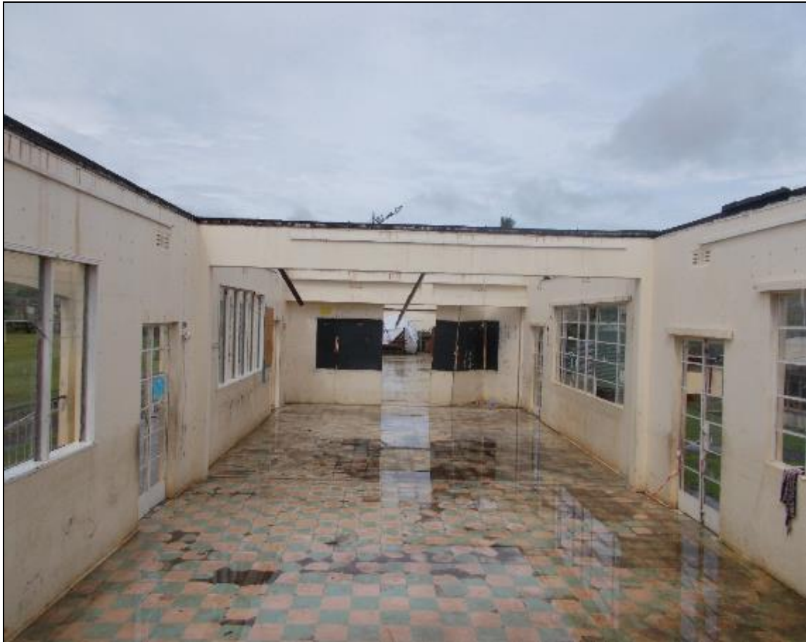
Photo 8 :View of water logged floor and blown off roof
