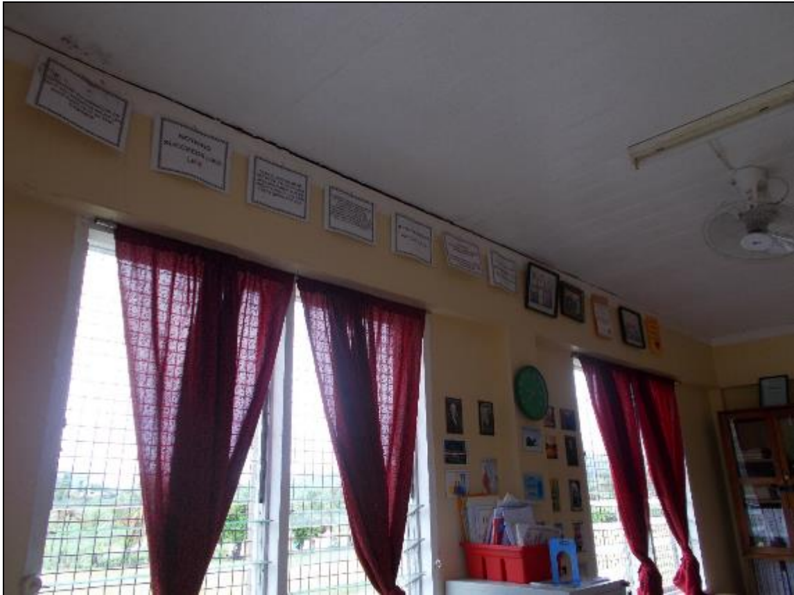
Photo 5: View of water damaged ceiling.
