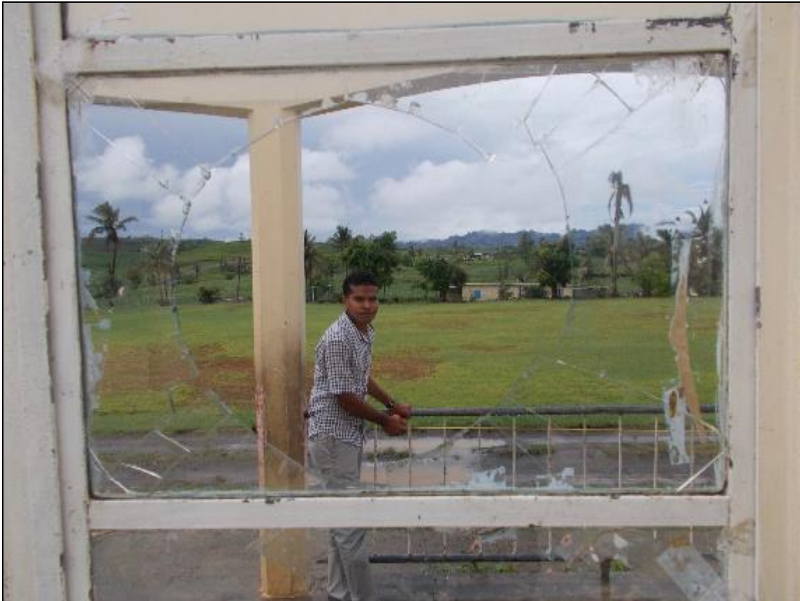
Photo 10: Damaged glazing on casement window.
