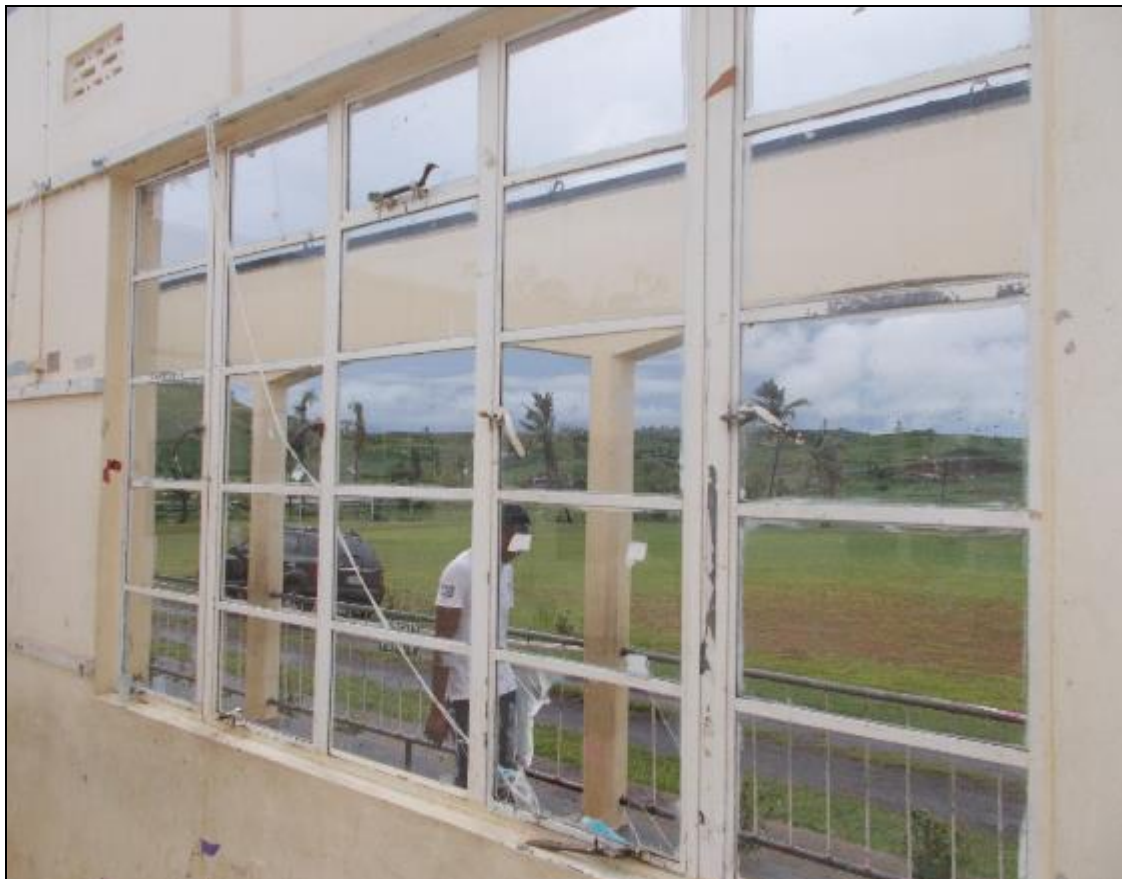
Photo 11: View of damaged casement window
