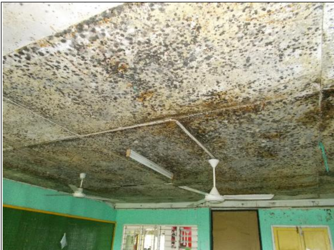
Photo 6: Water damaged ceiling under timber floor.
