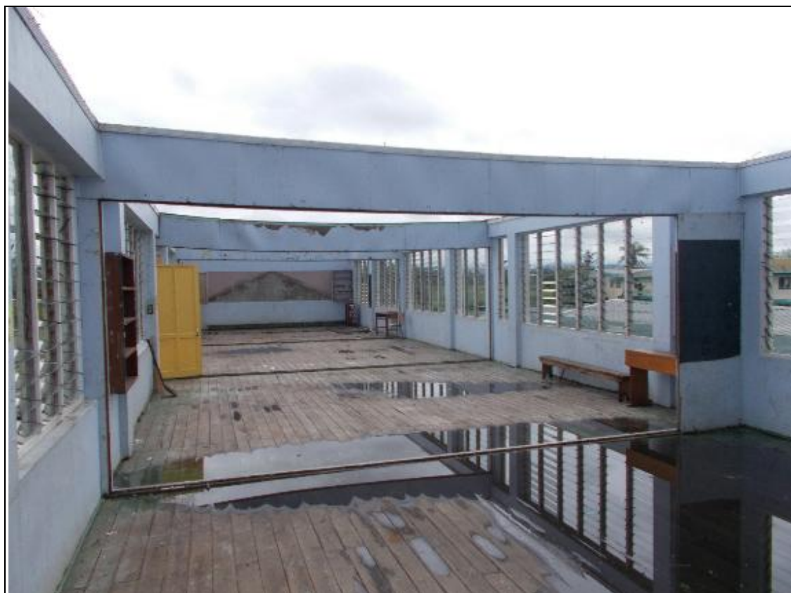
Photo 4: Completely blown off roof and water ponding on timber floor.
