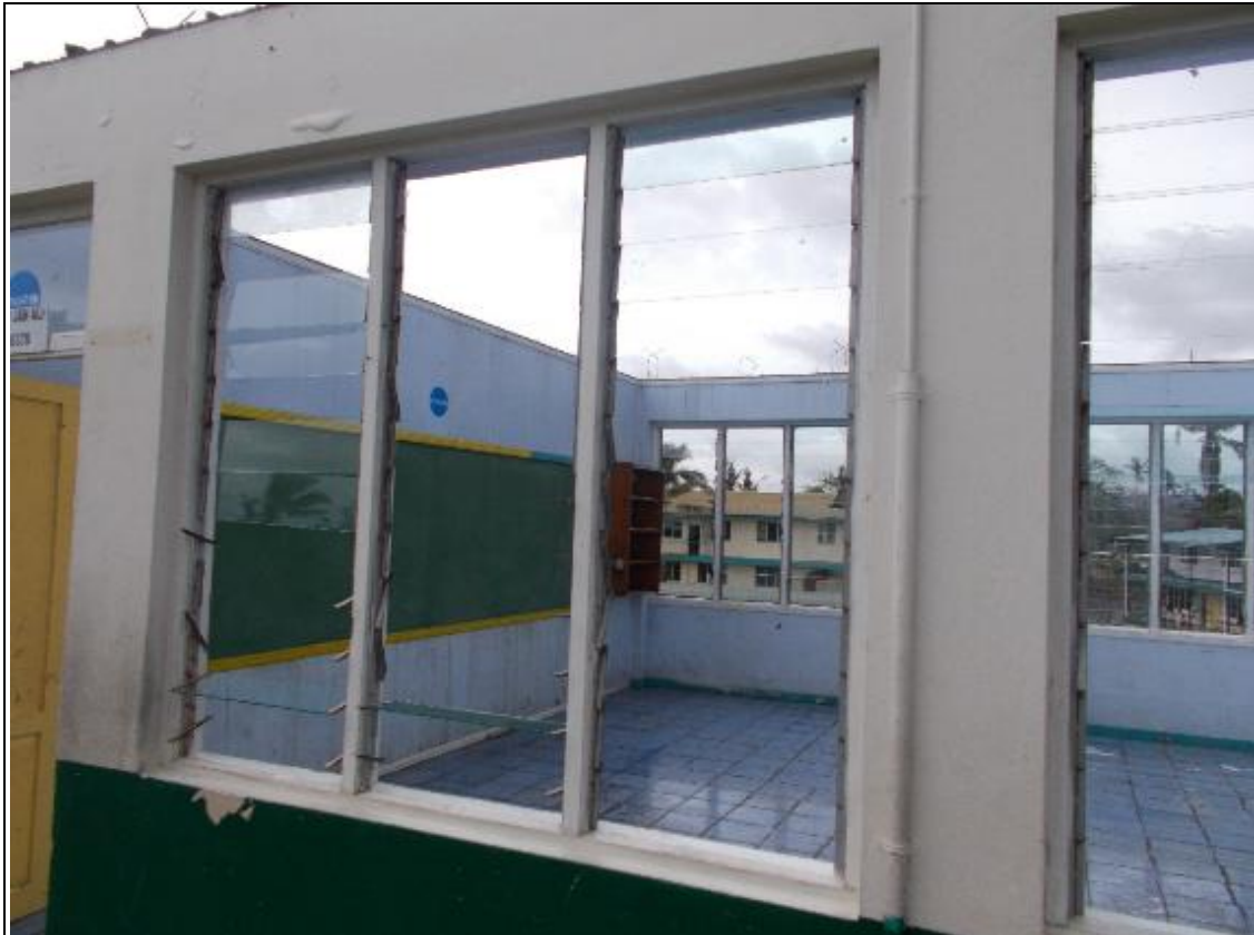
Photo 5: Broken louvers on windows
