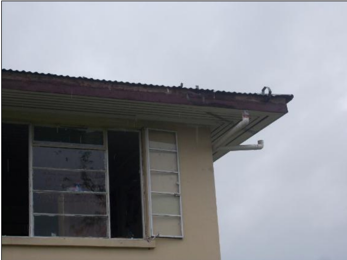
Photo 5: Showing TypicalAwning Windows / Damaged Gutters
