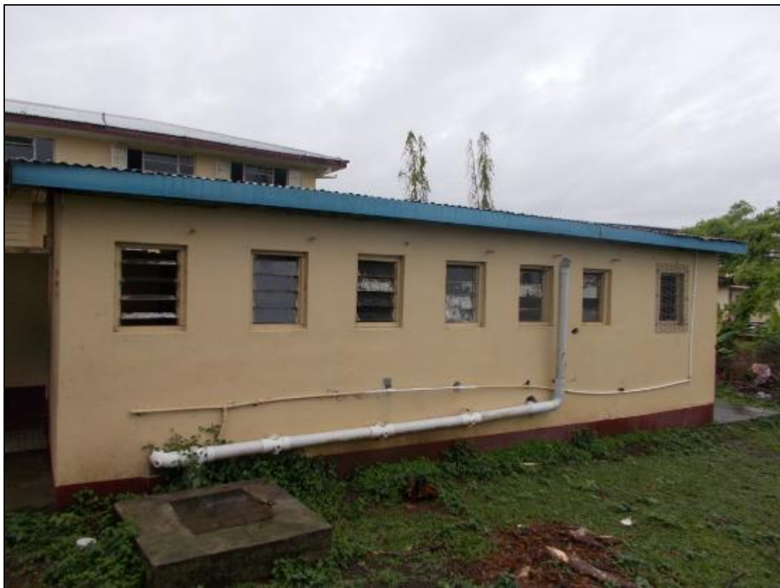
Photo 15: Typical Minor damages to Toilet Plumbing
