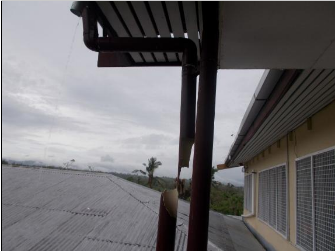
Photo 3: Roof view/Damaged downpipe
