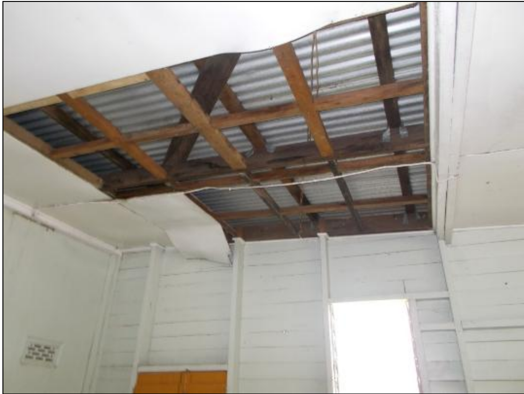
Photo 9: Showing Hall ceiling boards blown off
