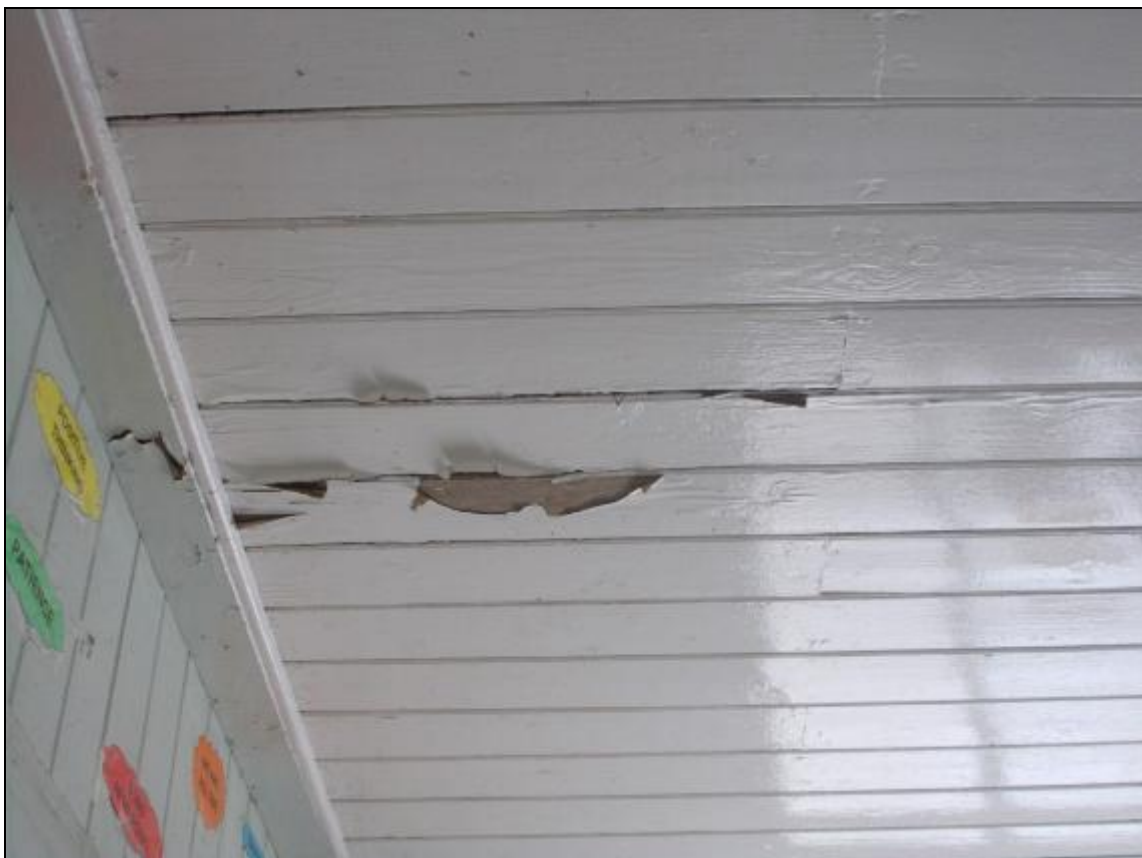
Photo 6: Showing typical water damaged ceiling
