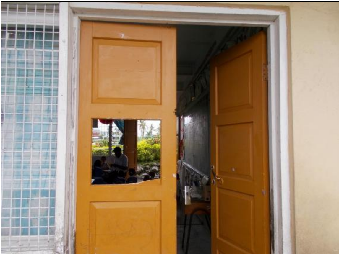
Photo 4: Showing Damaged door leaf
