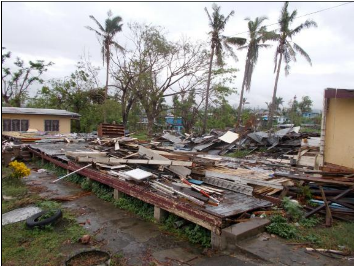
Photo 12: Total destruction of Building 3-Kindergarten
