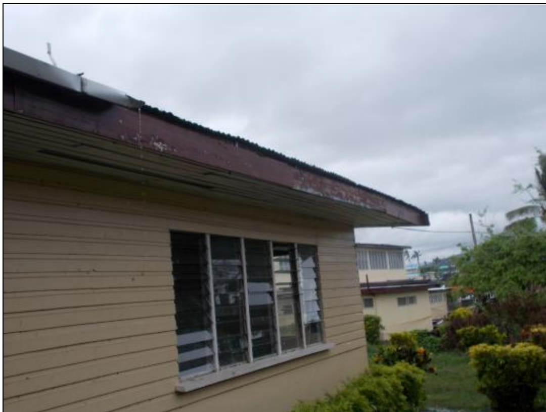
Photo 10: Showing typical Windows /Blown off gutters
