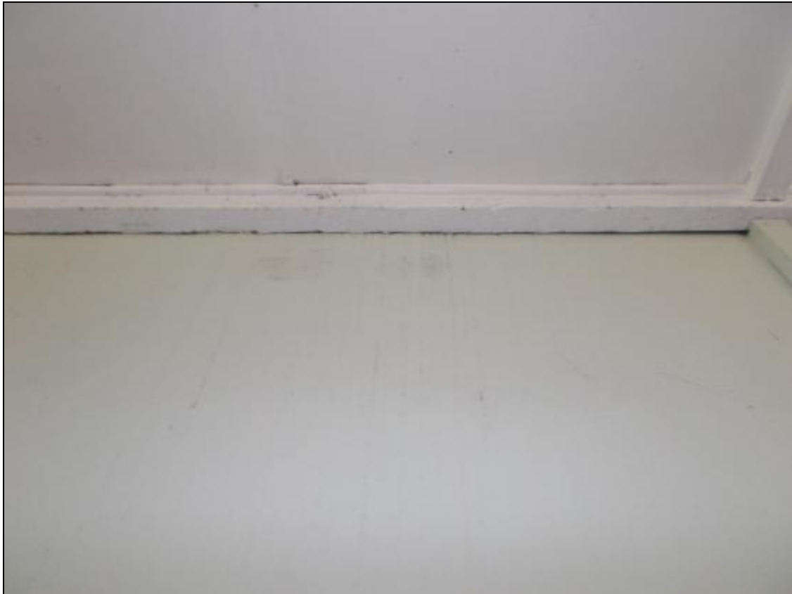
Photo 11: Showing water leak stains
