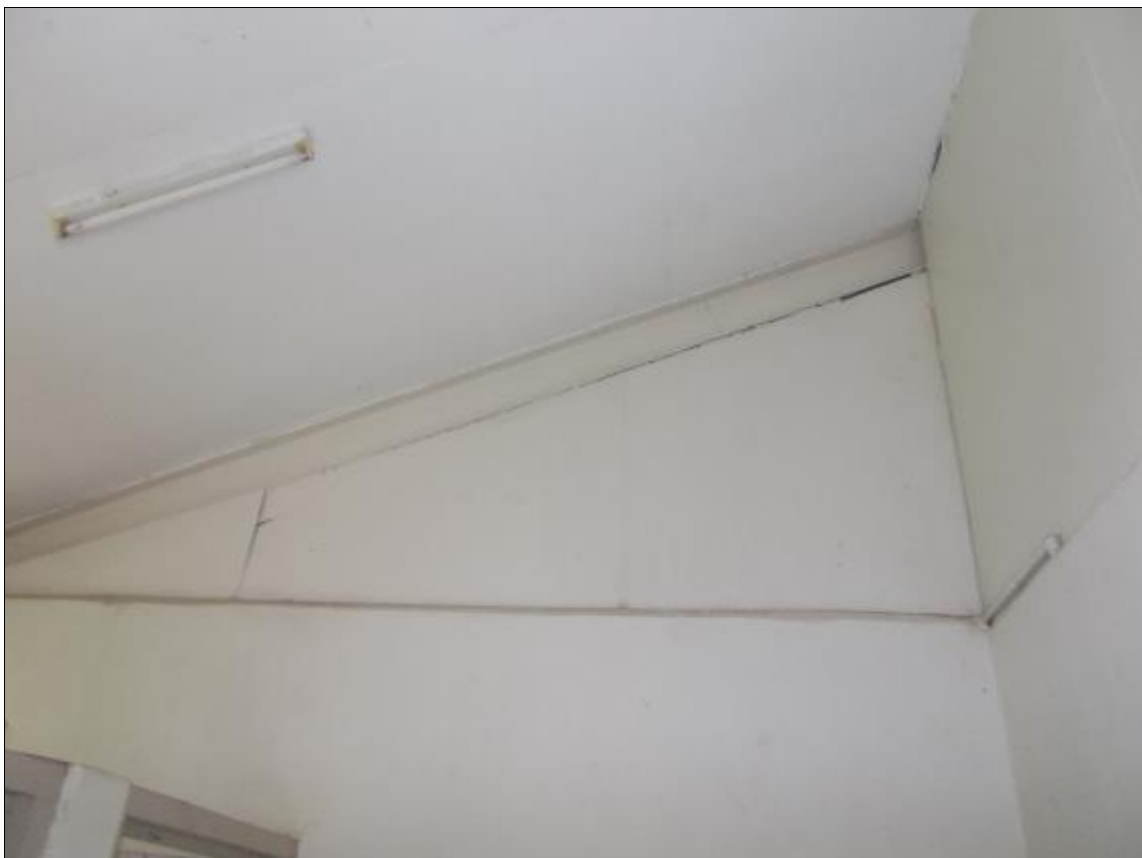
Photo 6: View of Interior Ceiling – Water Damage
