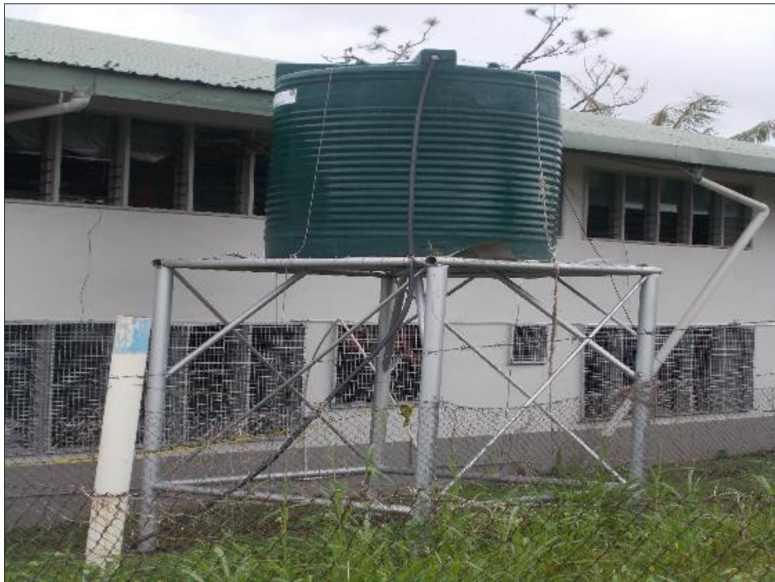
Photo 11: Rotomold Tank on Platform – Damage to plumbing
