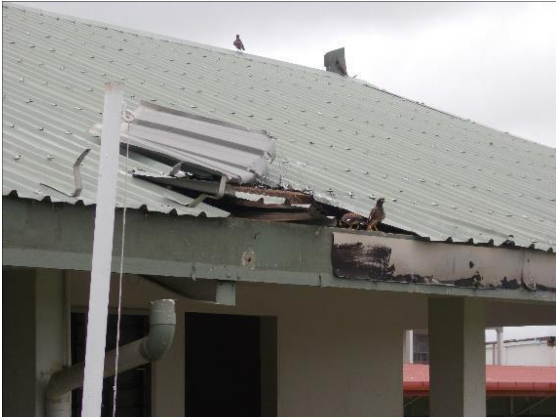
Photo 7: View of Roof – Damage to Cladding/Gutters and Flashings.
