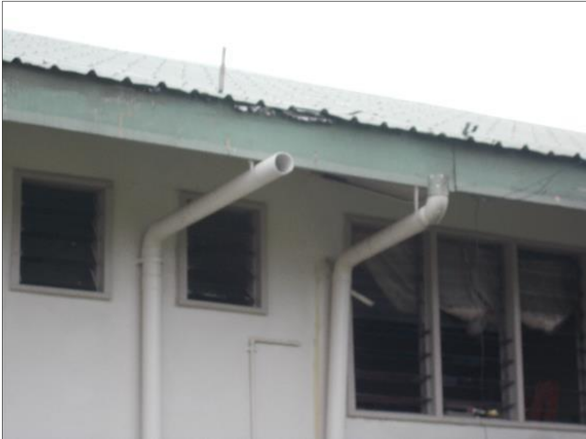
Photo 5: View of unshuttered windows/damaged plumbing
