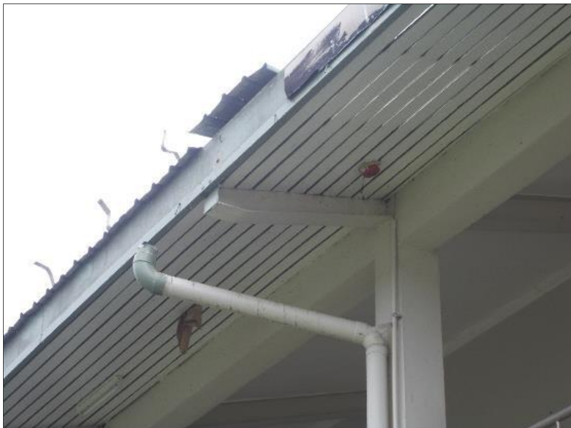
Photo 8: Blown out gutters
