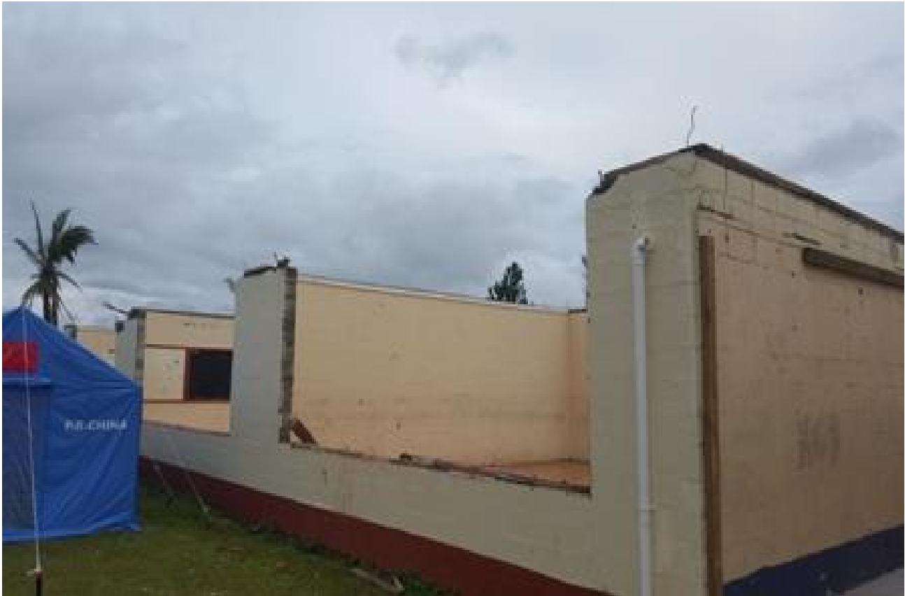
Photo 5: Fallen Wall of the School Block
