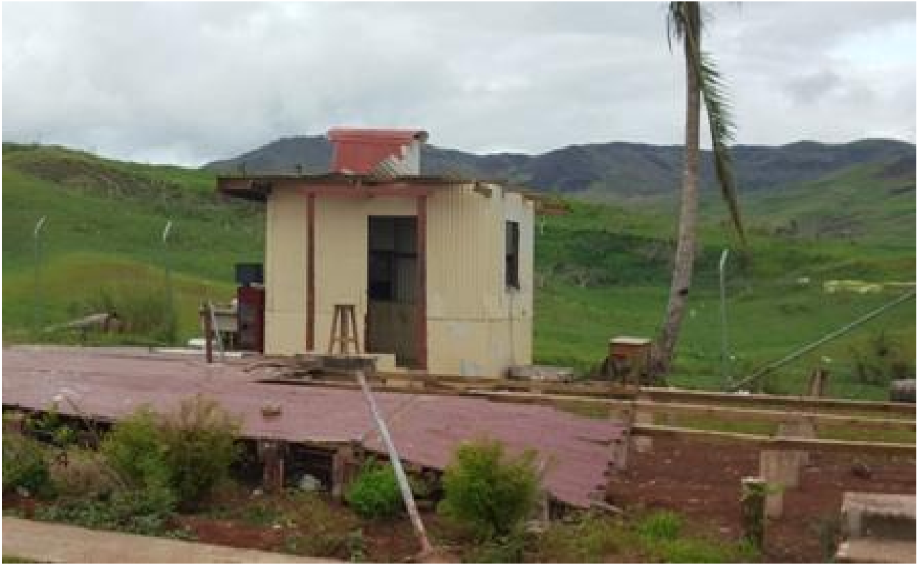
Photo 3: View of 100% Damaged Building
