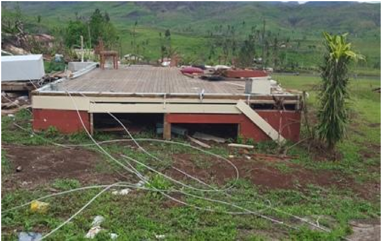
Photo 7: View of the 100% Damaged Teachers Quarters
