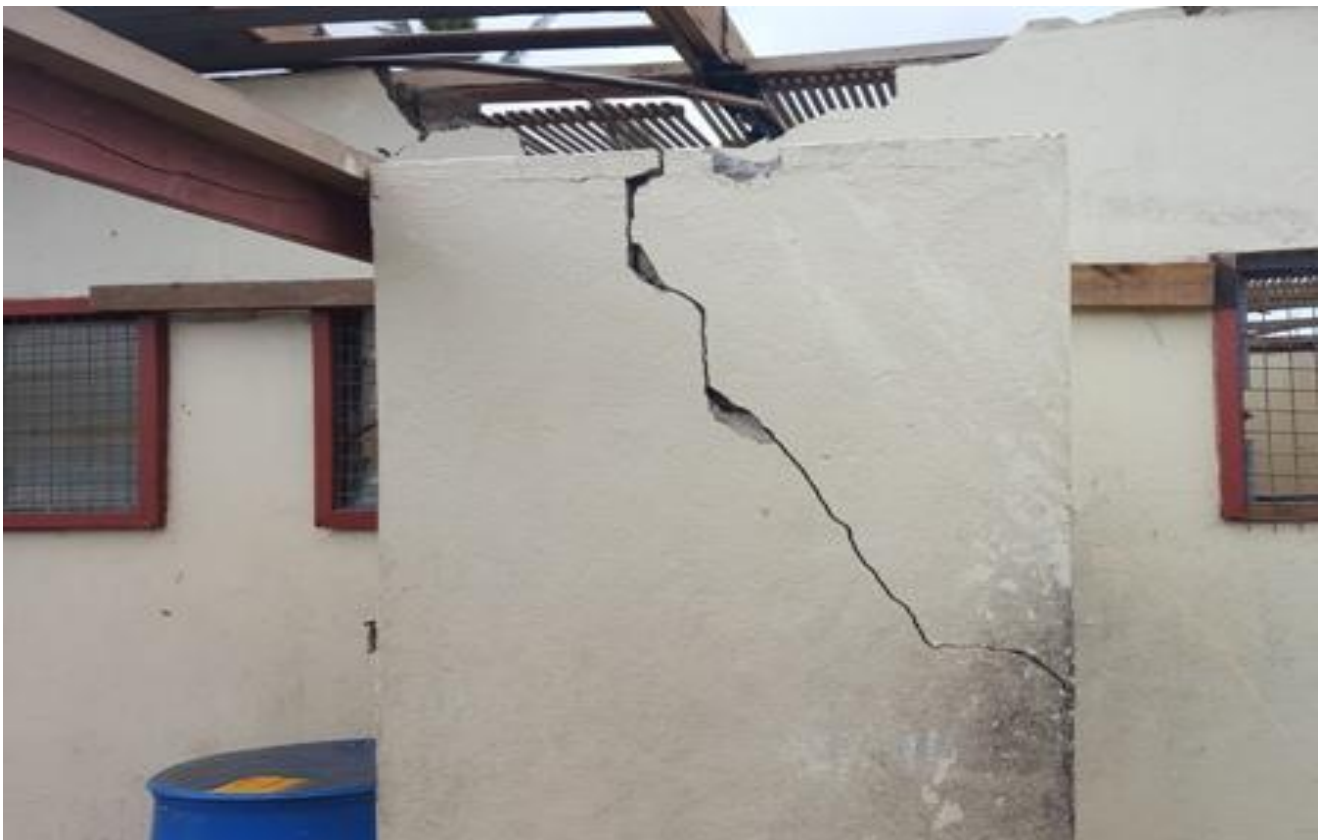
Photo 9: View of the Crack in Toilet Block
