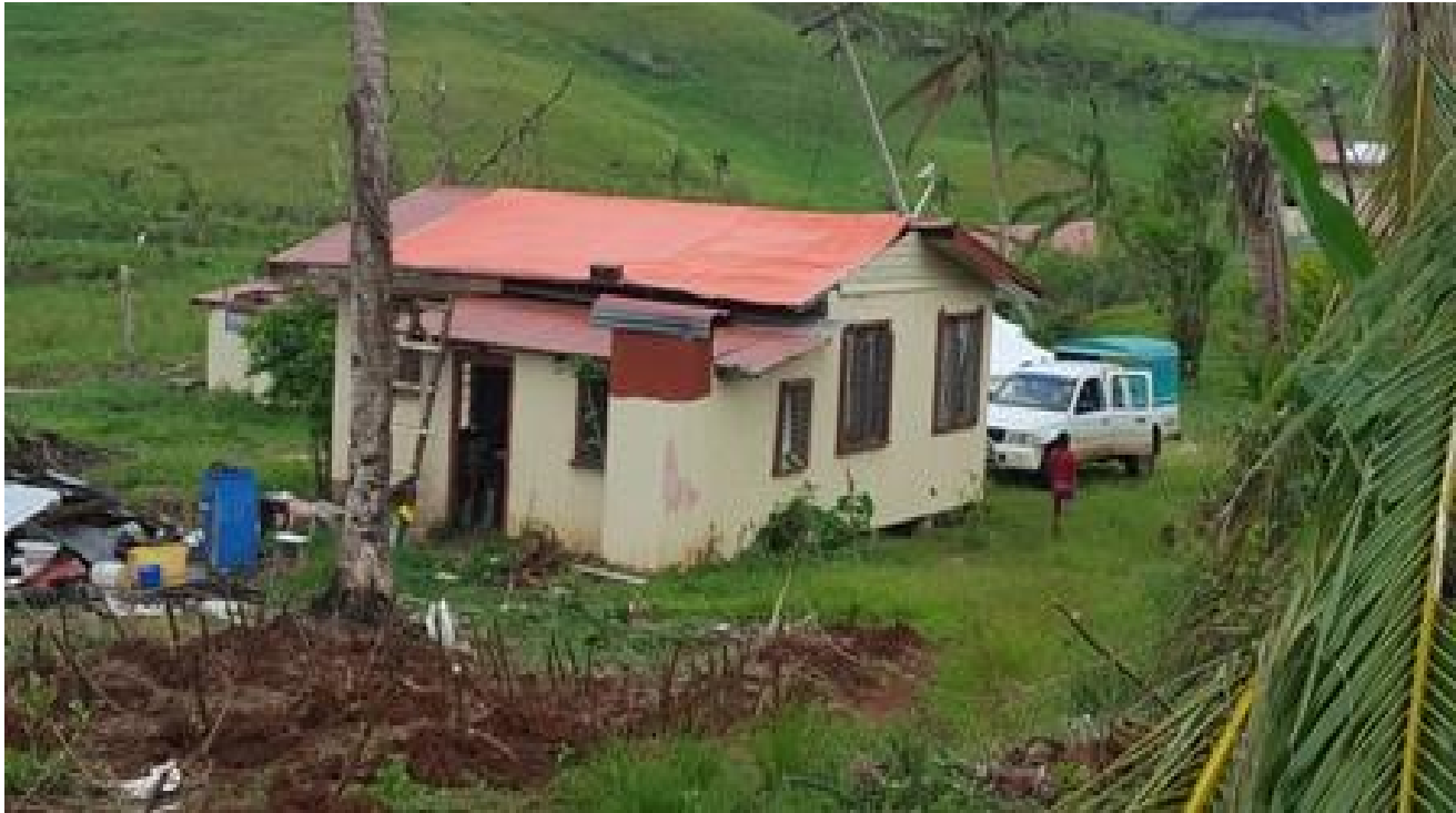
Photo 6: View of the Teachers Quarters with Damaged Roof
