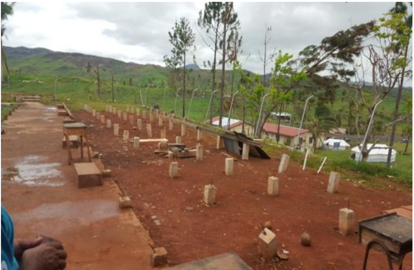
Photo 2: View 100% damaged Building
