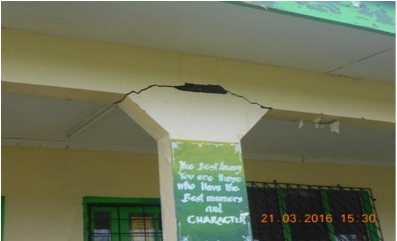
Photo 5: Column Crack View
