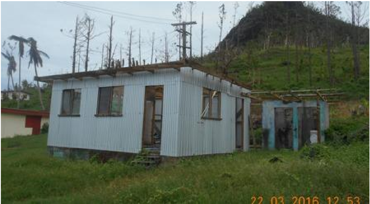
Photo 3: View of the Damaged Teachers Quarters
