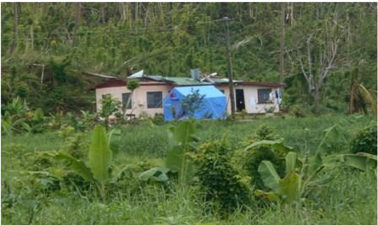
Photo 4: View of the Damaged Teacher Quarters.
