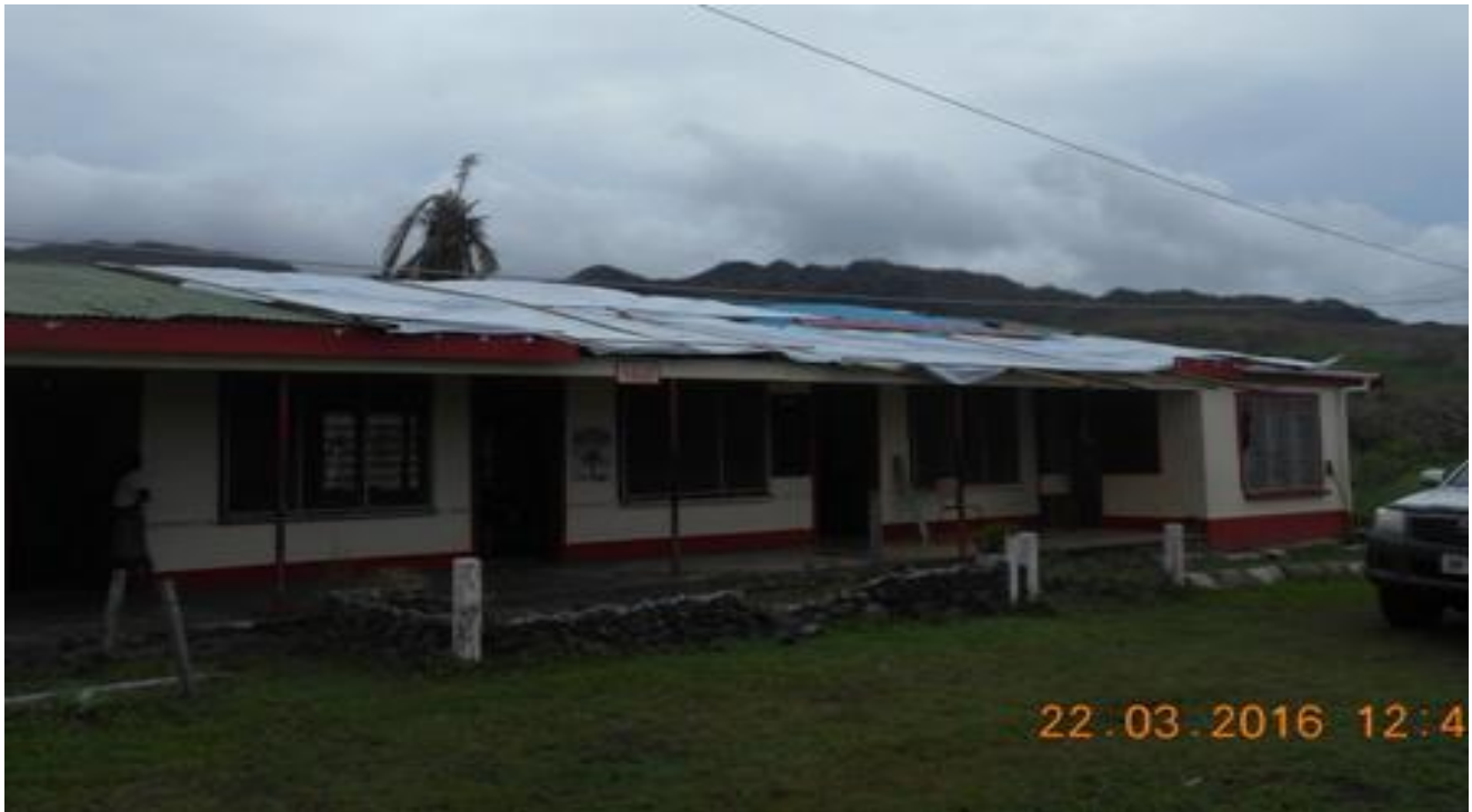
Photo 1: View of the School Building with Damaged Roof
