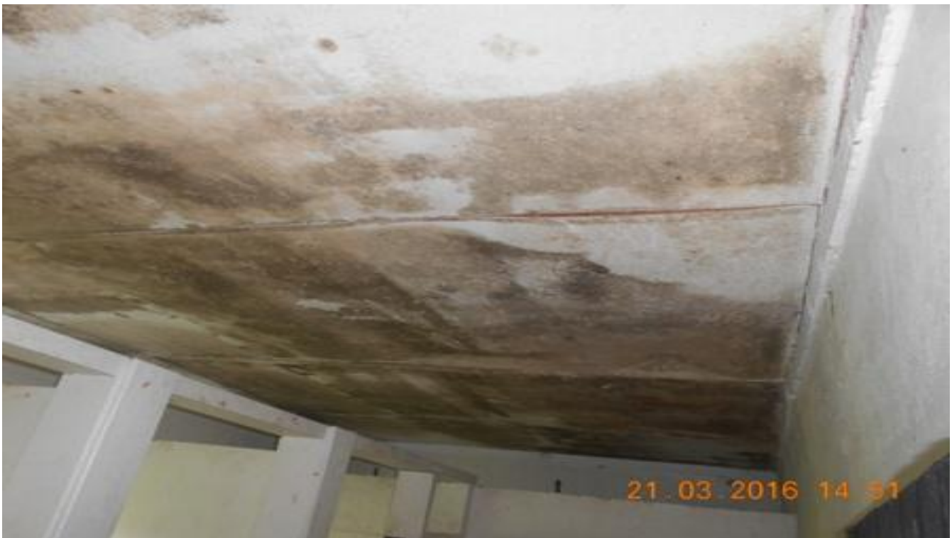
Photo 11: Water Damaged Ceiling
