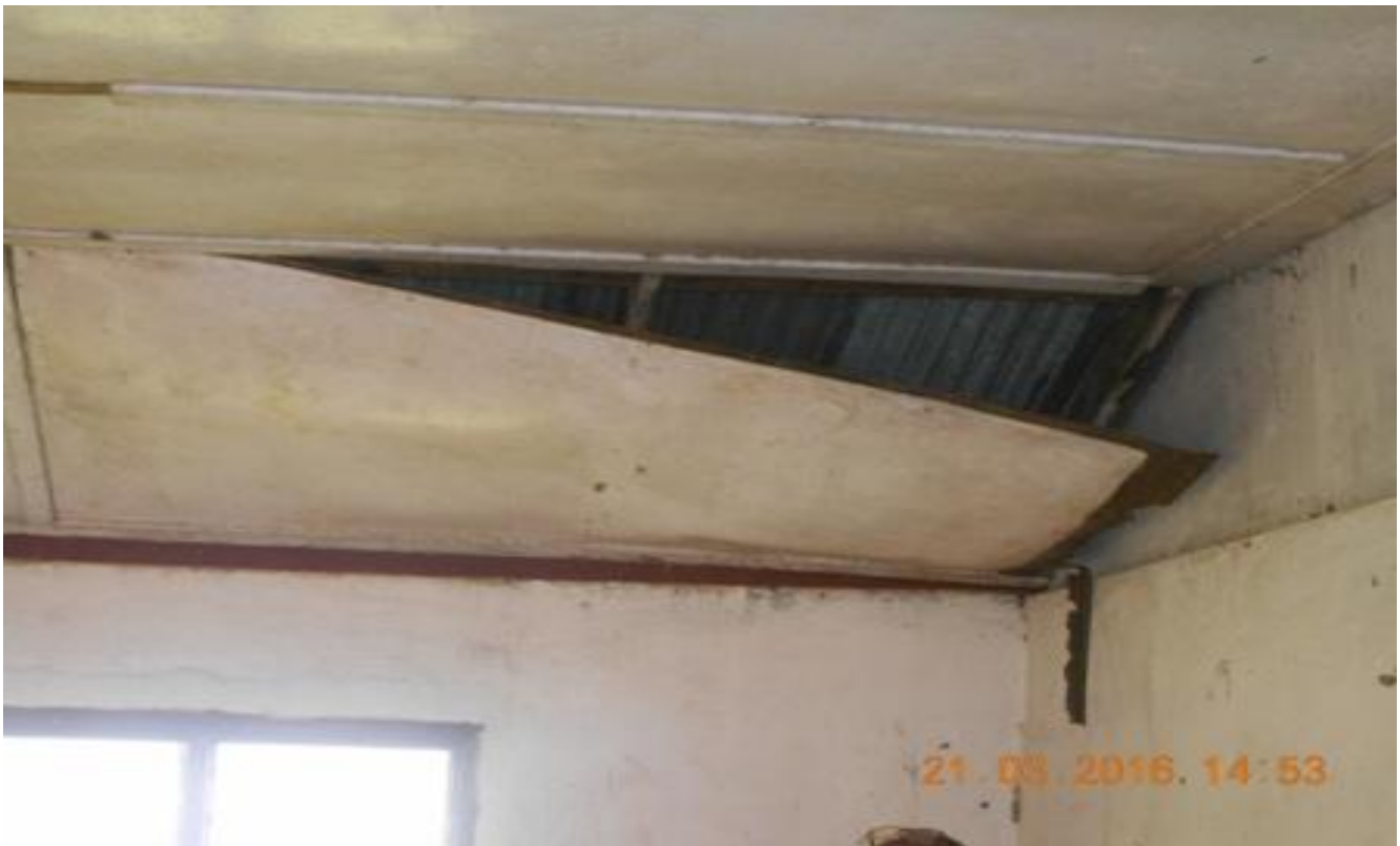
Photo 8: View of the Water Damaged Ceiling
