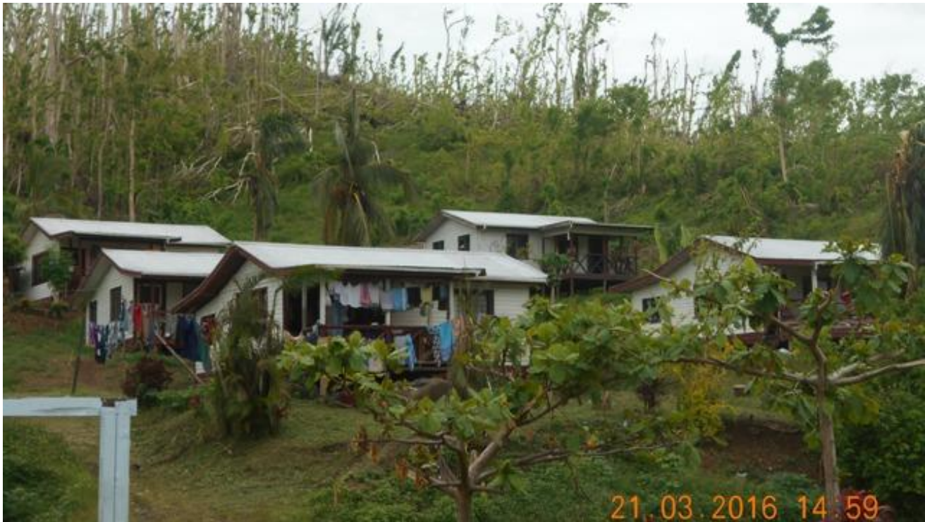
Photo 12: Showing Overall View of Staff Quarters- Very Minor Damage- Guttering, Downpipes ,Flashings
