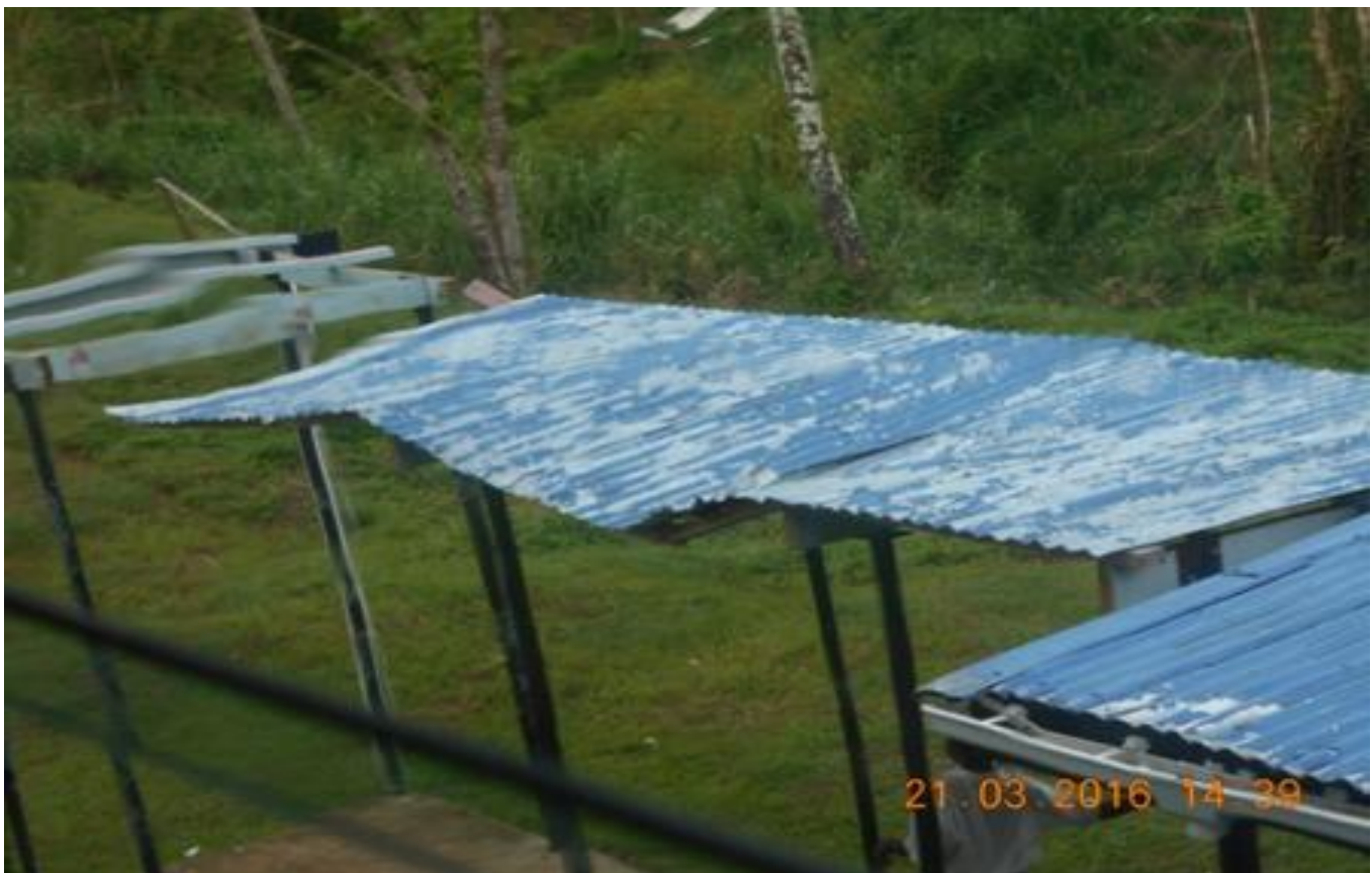
Photo 14: Showing Damaged Walkway
