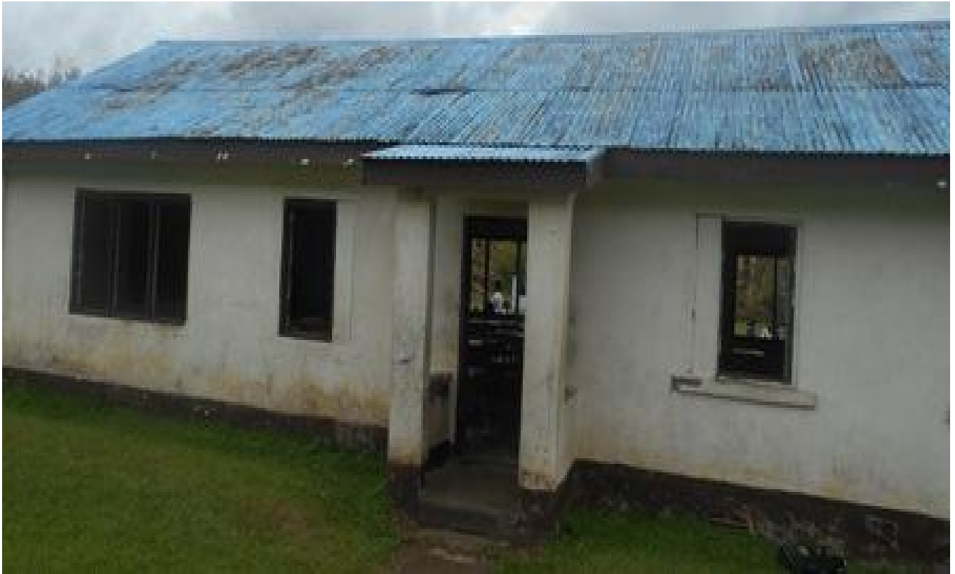
Photo 7: View of Damaged Roof
