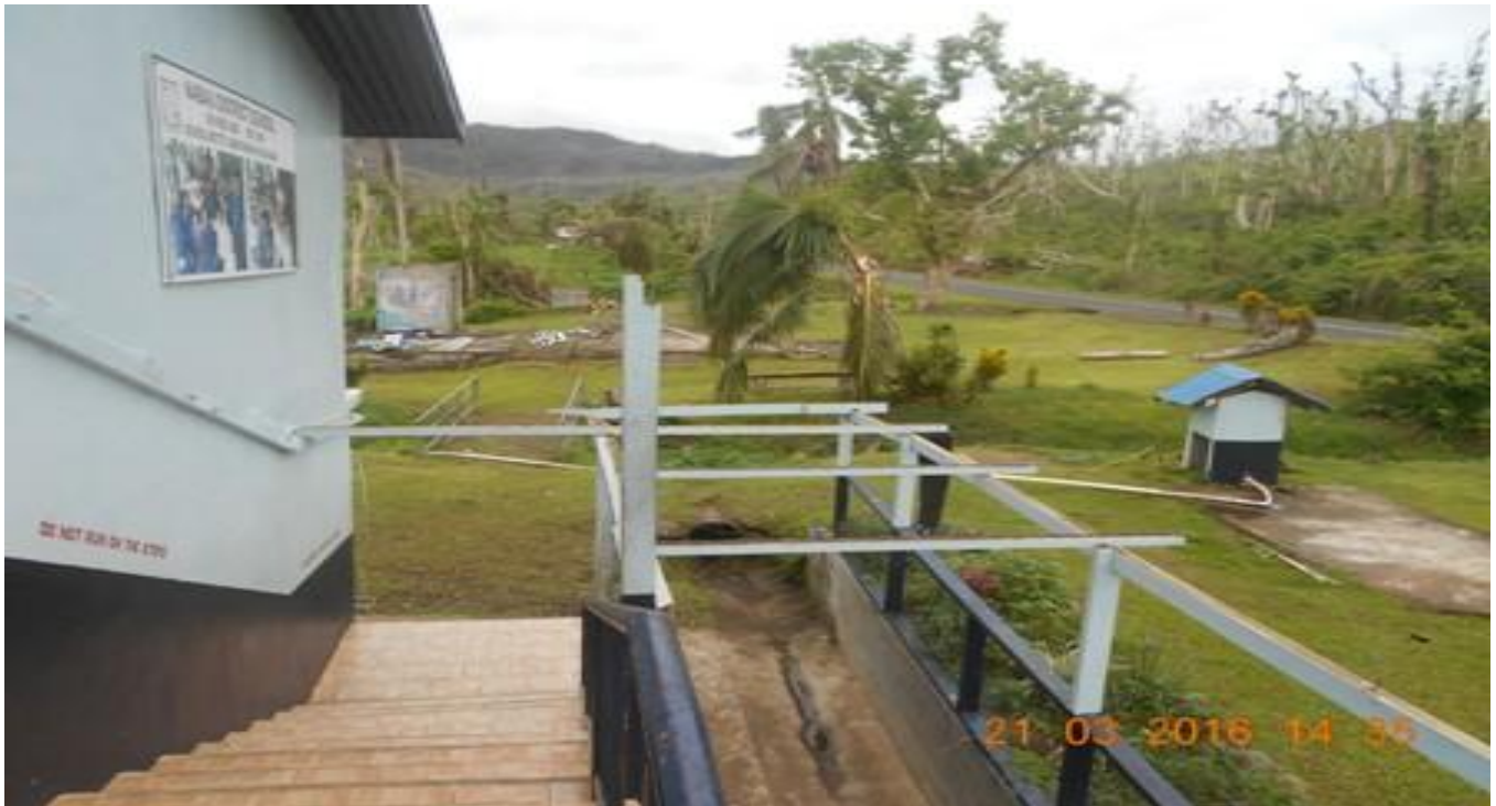
Photo 13: Showing Damaged Walkway
