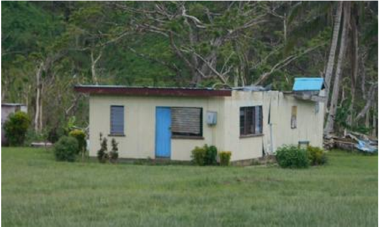
Photo 6: View of Corrugated Teachers Quarters with Damaged Roof
