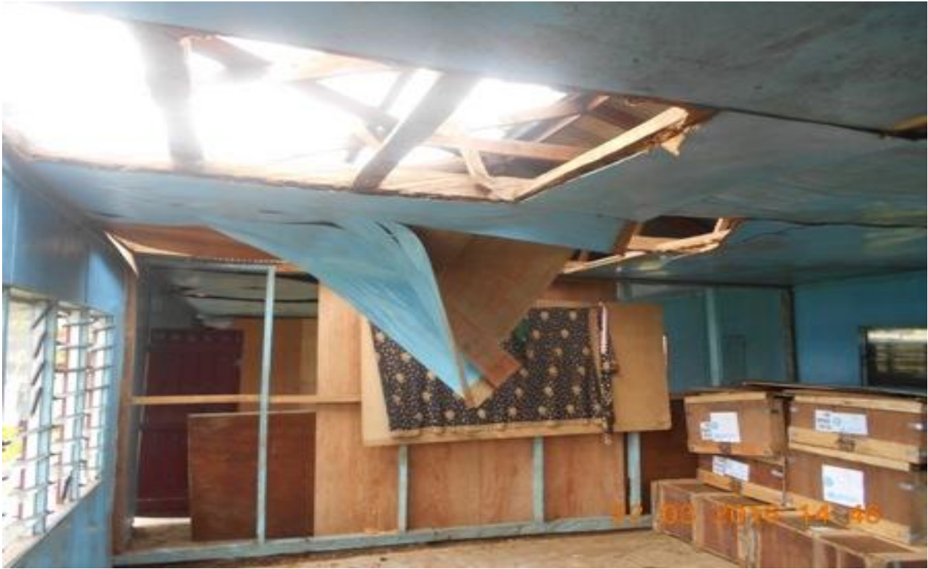
Photo 5: Overall View of Water Damaged Ceiling
