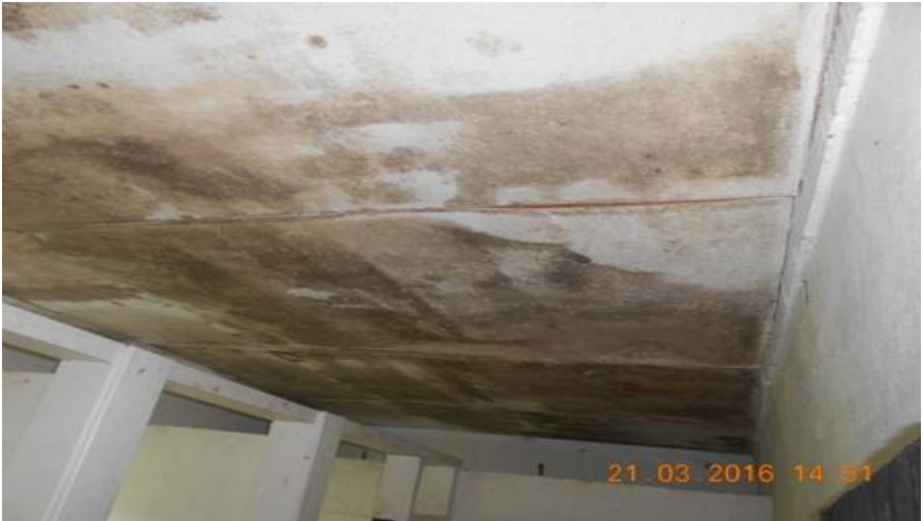
Photo 11: Water Damaged Ceiling
