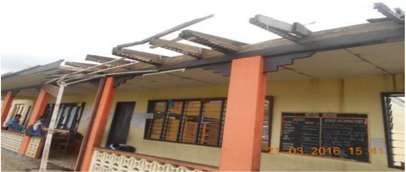
Photo 1: Verandah Portion has been blown away
