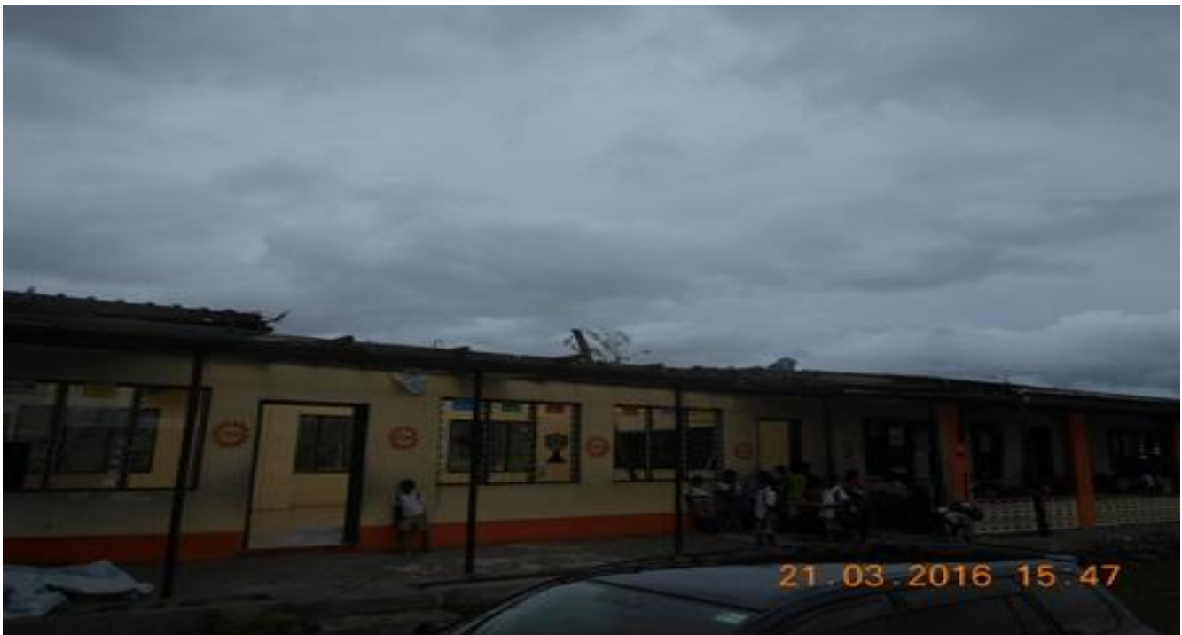
Photo 2: View of the Damaged Building
