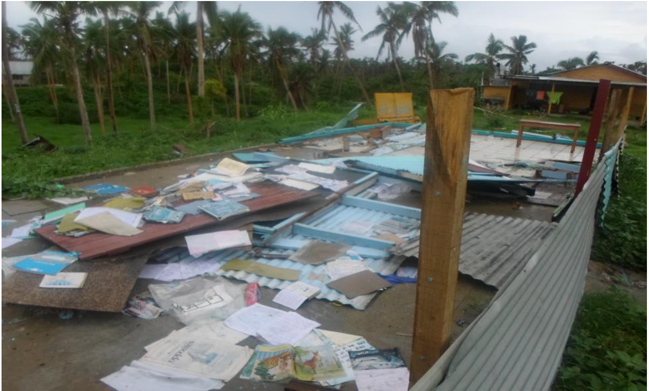
Photo 5: Overall building photos that totally blown away
