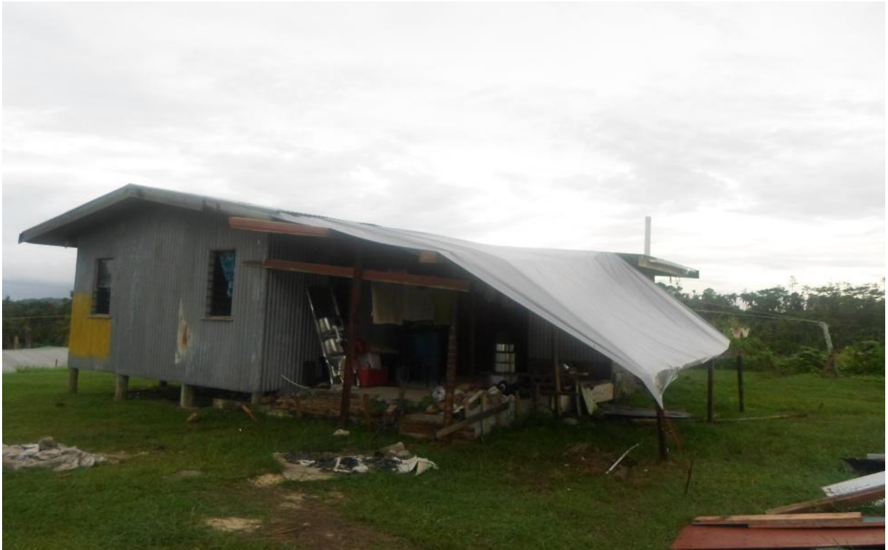
Photo 9: Overall building photos for partly damaged staff quarters
