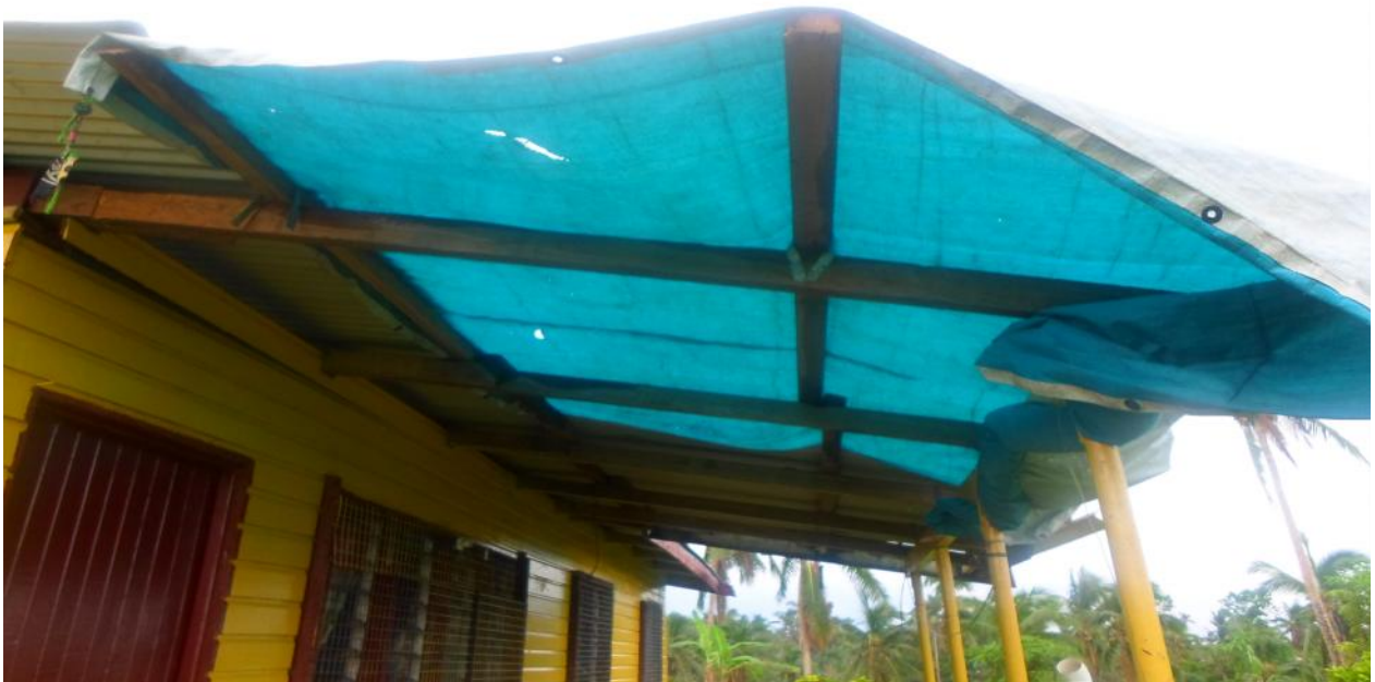
Photo 8: View of verandah the that was blown away
