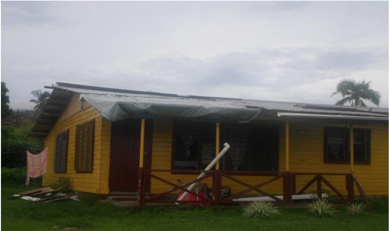
Photo 7: Overall building photos that totally blown away
