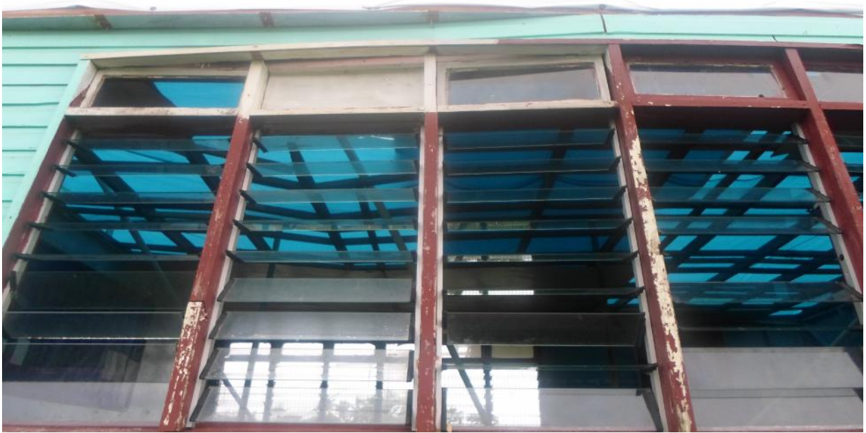
Photo 3: Enlarge view of the damage walls
