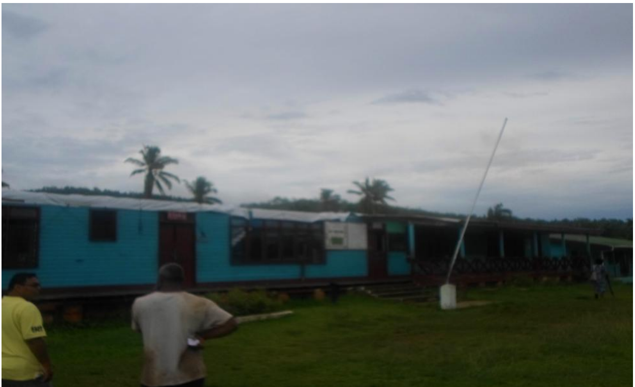
Photo 2: Overall frontage view of the building that is damaged
