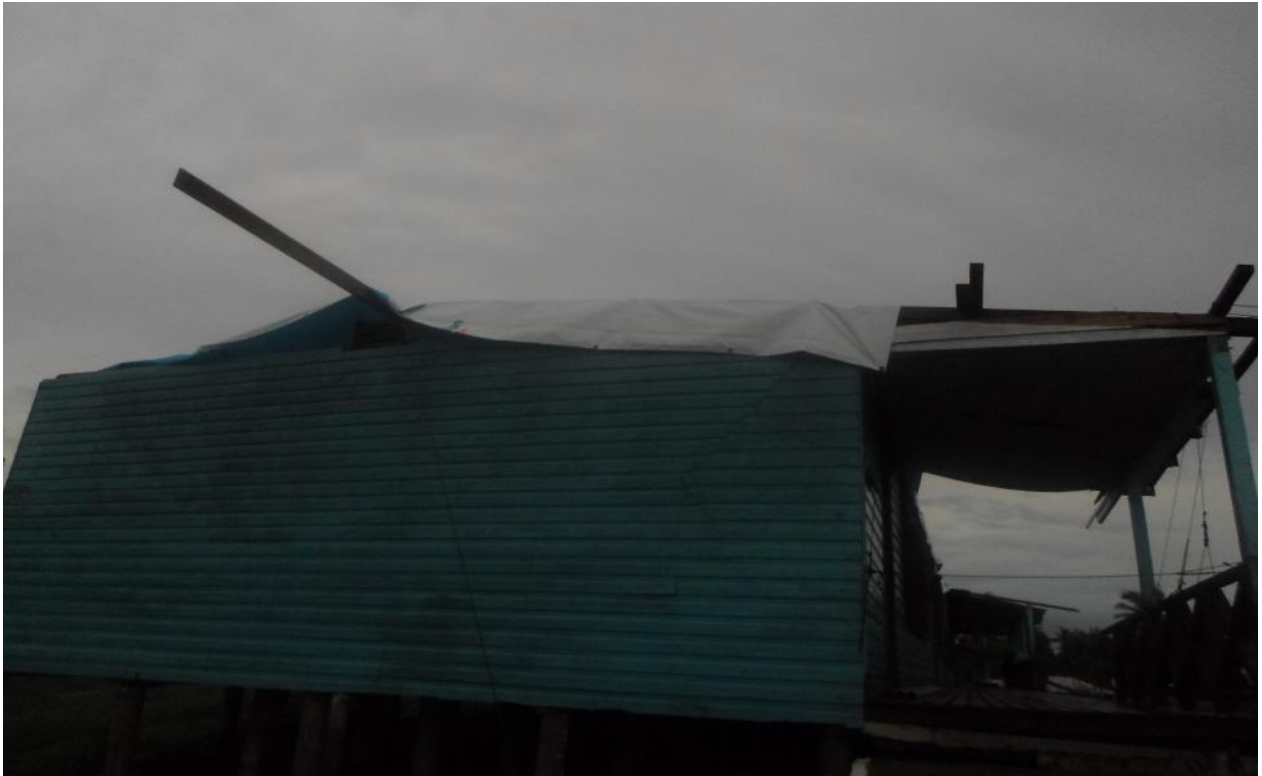
Photo 1: Side view of the building that is damaged
