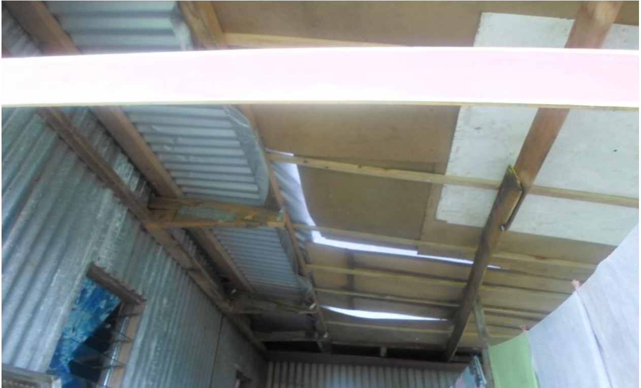
Photo 10: Enlarge view of the part that was blown away
