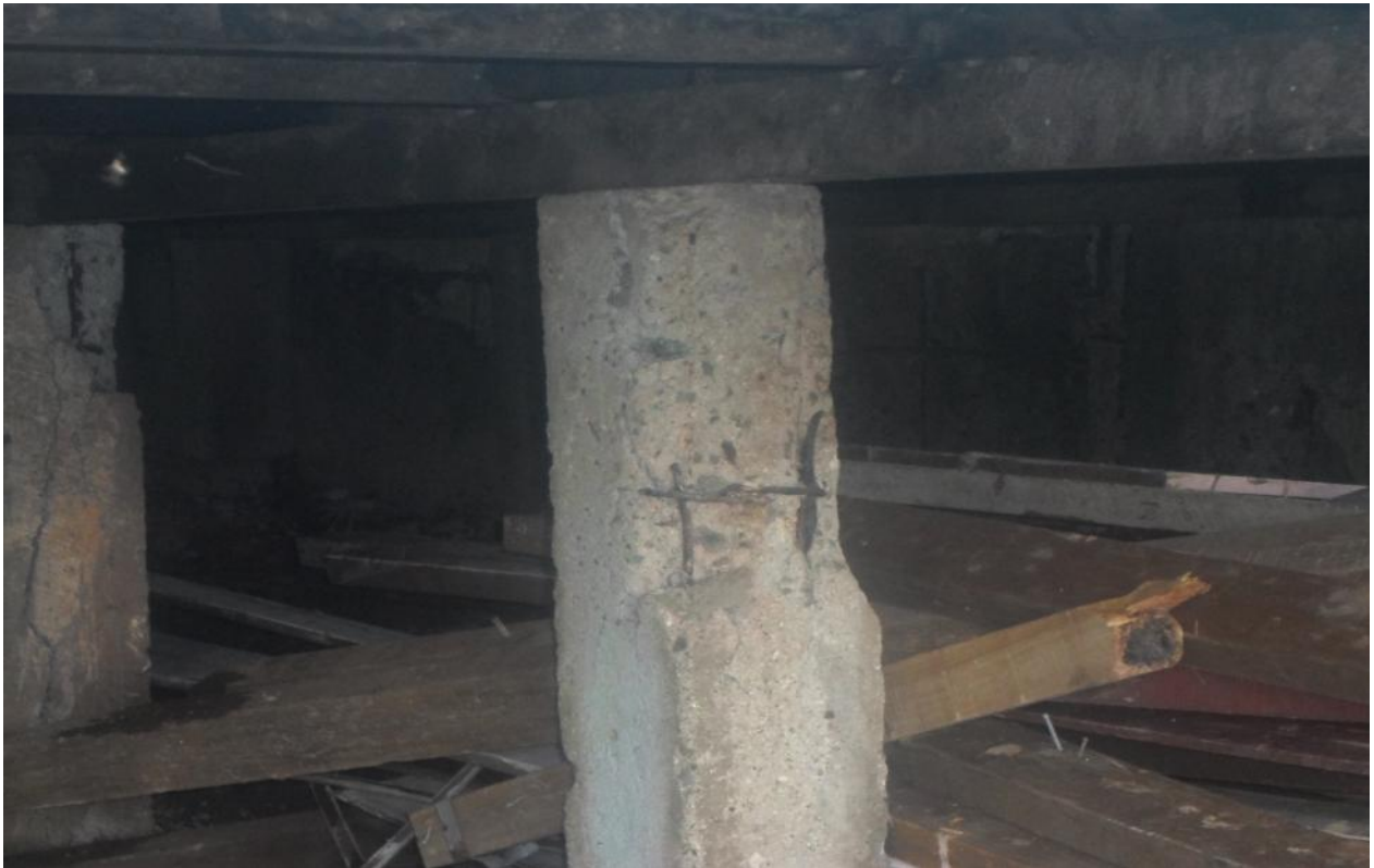
Photo 4: Damaged concrete post
