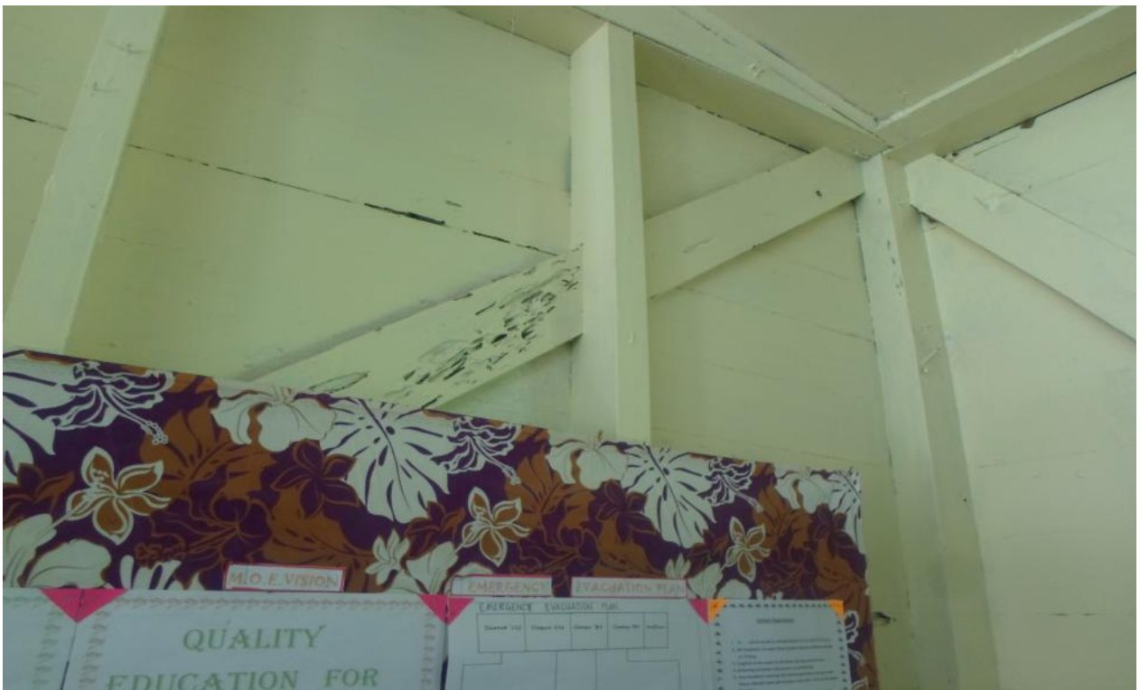
Photo 2: inside wall of the building that is damaged
