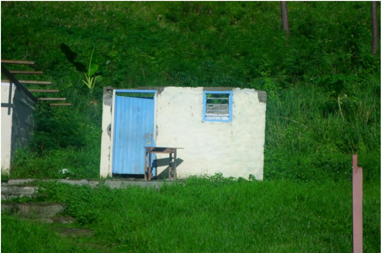
Photo 4: Toilet block that was damaged in cyclone
