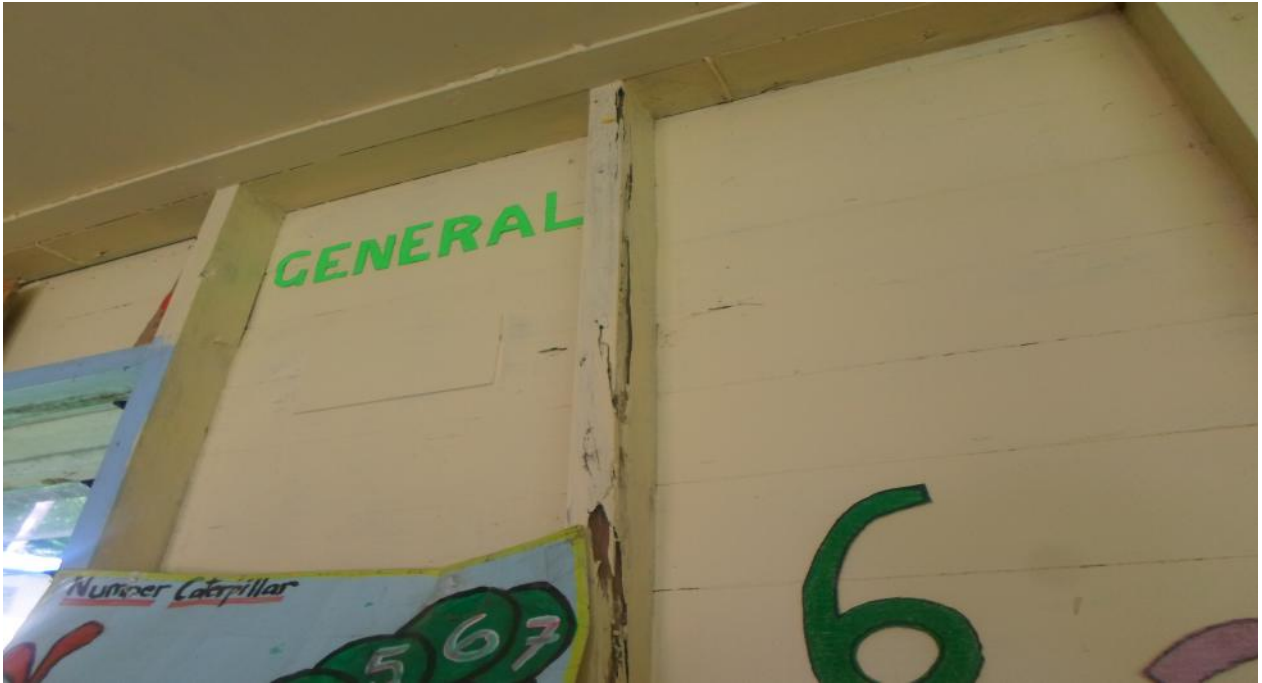
Photo 3: Inside members of wall of the building that was damaged
