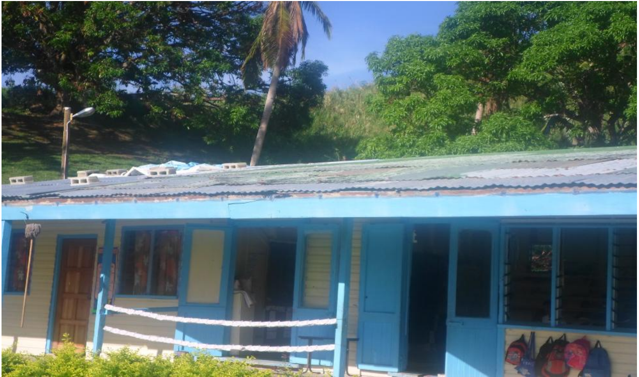
Photo 1: Side view of the building that is damaged
