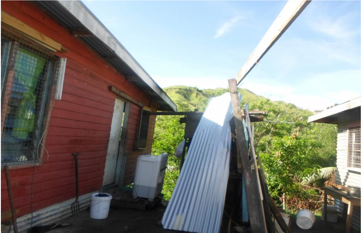
Photo 5: Outdoor kitchen for the staff quarters that was blown away
