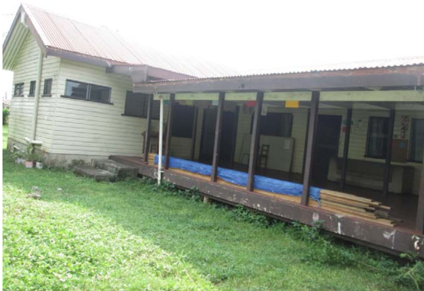
Photo 4: Rear View of Building 1- Showing Missing Guttering & Downpipes
