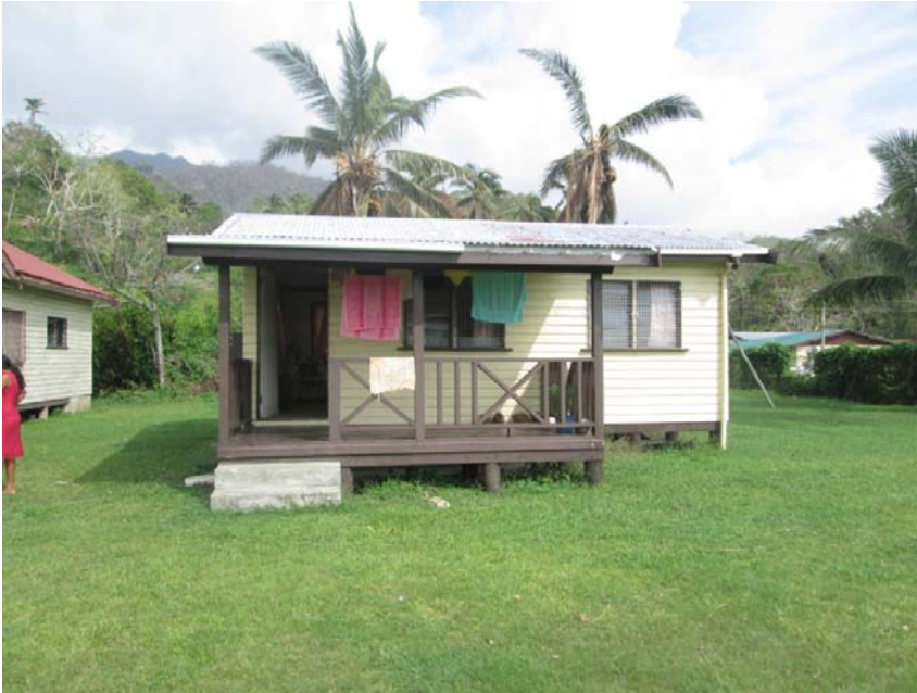
Photo 5: Front View of building 2 – Showing Damaged Guttering
