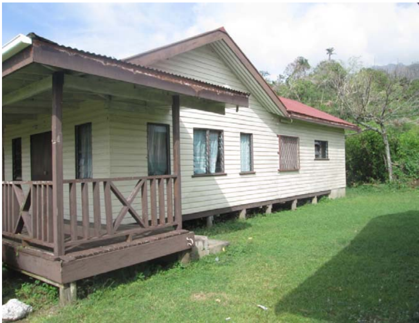
Photo 2: Side View of building 1- Showing Missing Flashing, Guttering & Deteriorated Fascia
