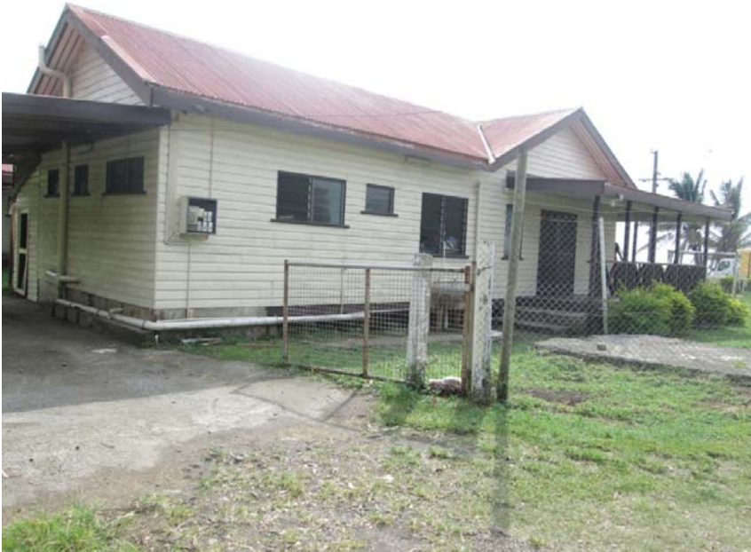
Photo 3: Side & Roof View of Building 1- Showing Missing Guttering
